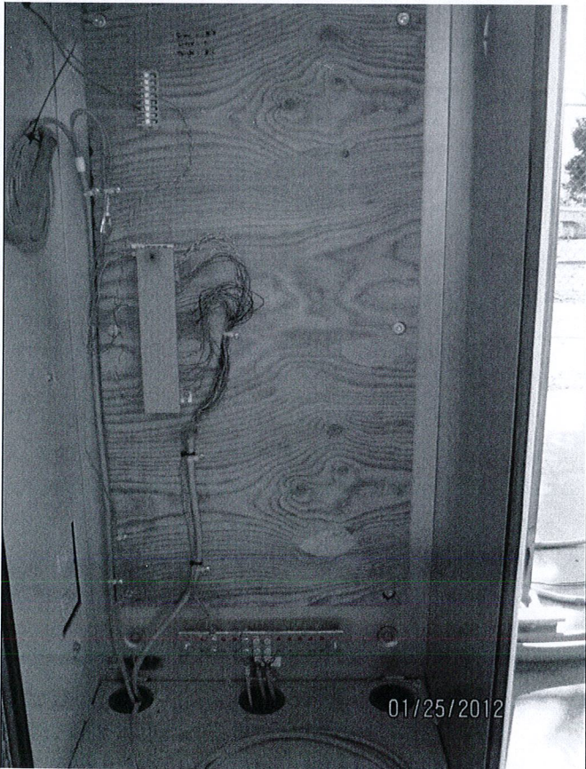
4 EXISTING TELCO CABINET
