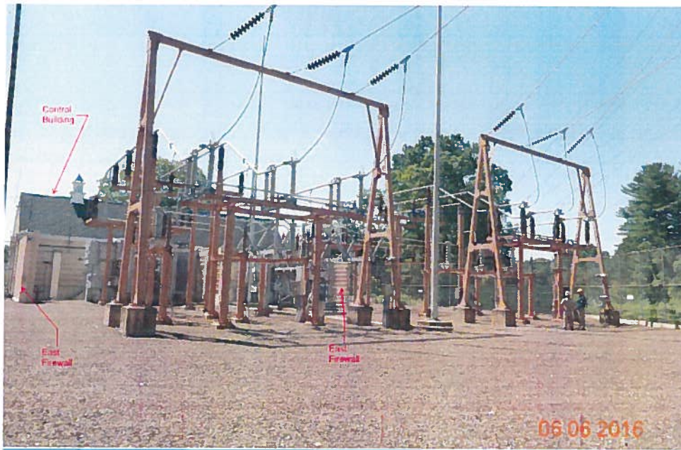
Trap Falls Substation looking South
