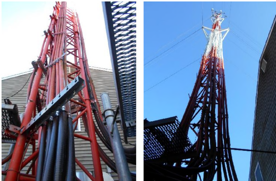
Photos of existing feed lines at tower.
