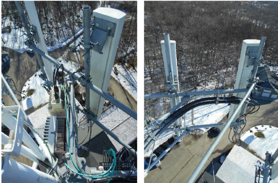
Photos of Verizon's typical existing equipment and mounts at 155'.
