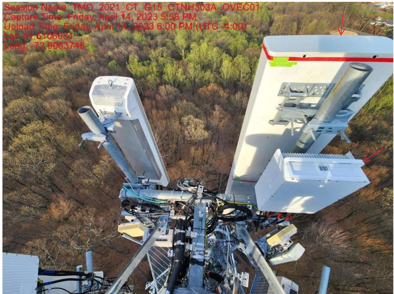
Alpha Sector: (1) New Antenna & (1) New RRH Mounted To Existing T-Arm Mount
