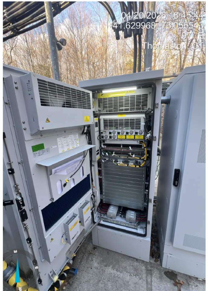
Self support cabinet installed on concrete pad
