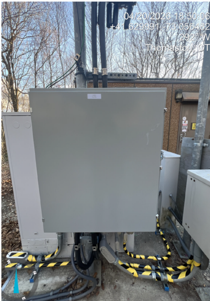
New slack box installed on unistrut frame
