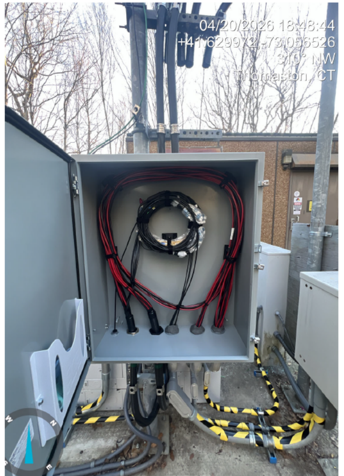
New slack box installed on unistrut frame
