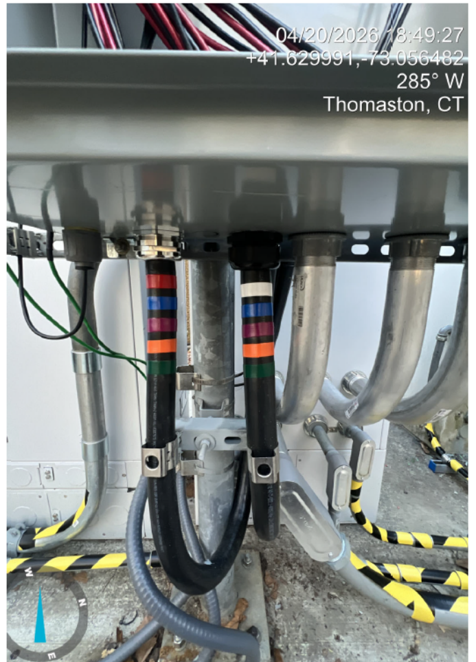
New connections at slack box
