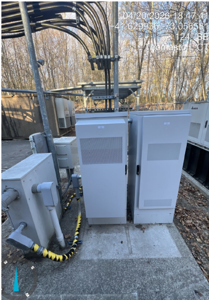
Self support cabinet installed on concrete pad
