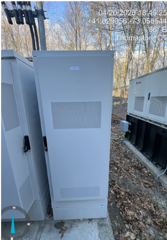
Battery cabinet installed on concrete pad
