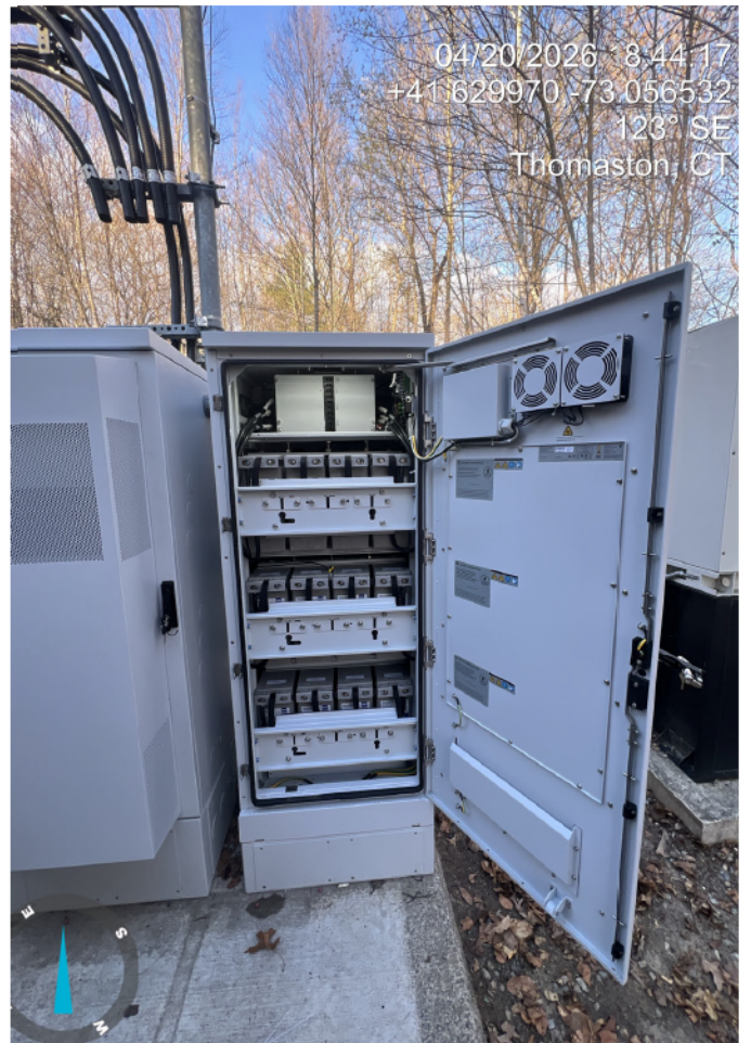
Battery cabinet installed on concrete pad
