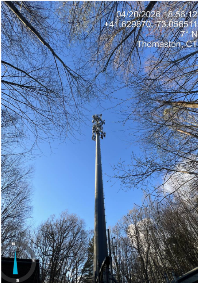
Overall view of installation
