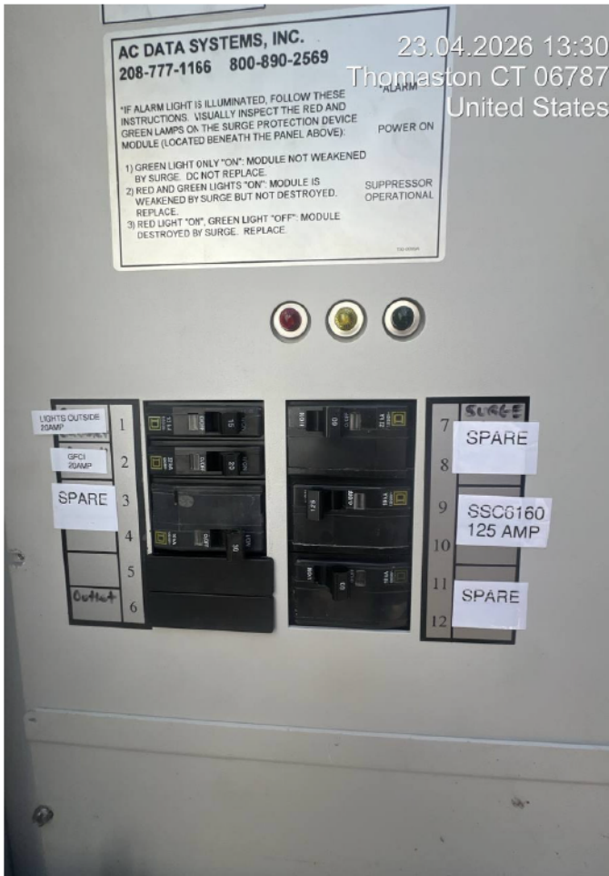
New breaker for 6160 cabinet
