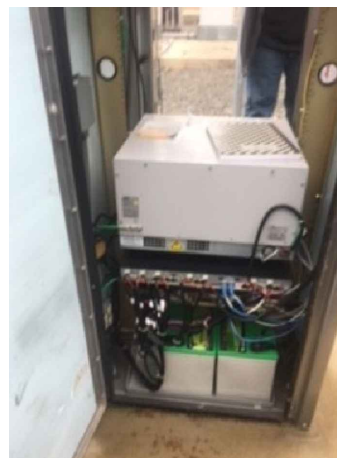
INSIDE CLEARWIRE CABINET
