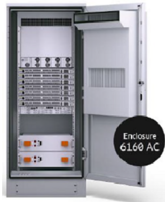
ERICSSON RBS6160 EQUIPMENT CABINET
