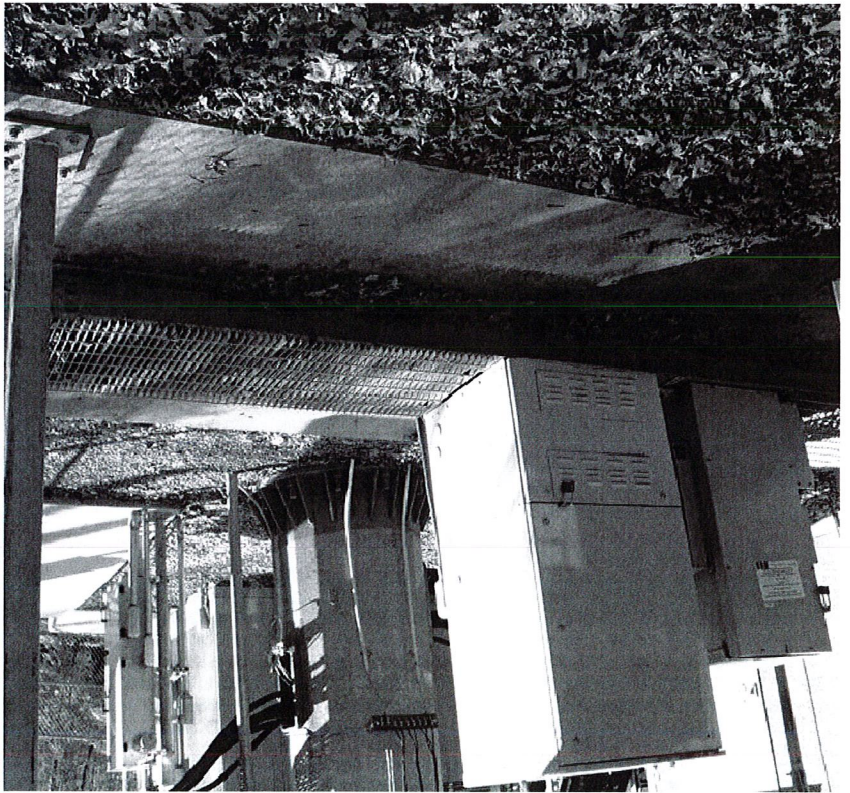
3 EXISTING EQUIPMENT AREA
