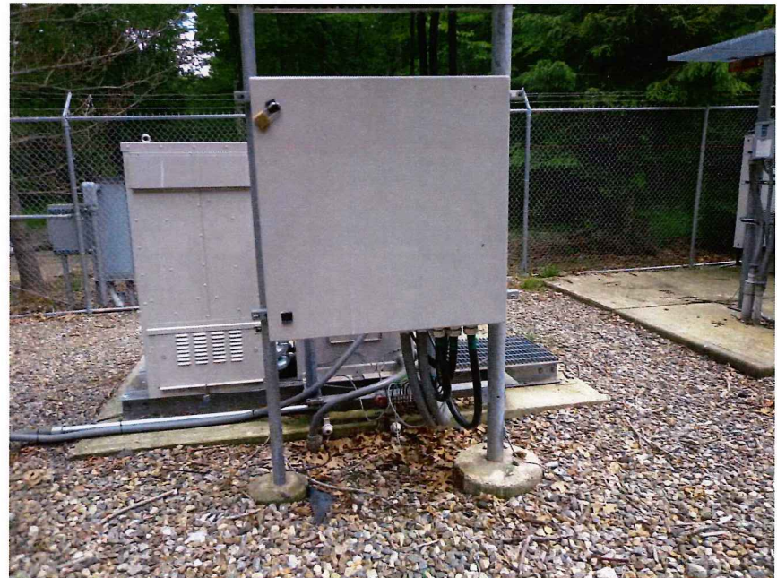
4 EXIST FIBER DISTRIBUTION BOX SCALE: NTS
