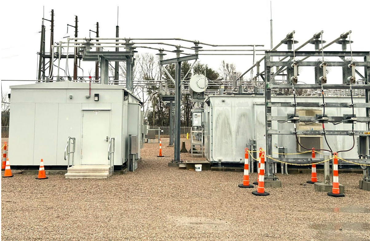
Figure 1 - New Switchgear (enclosure on the left)
