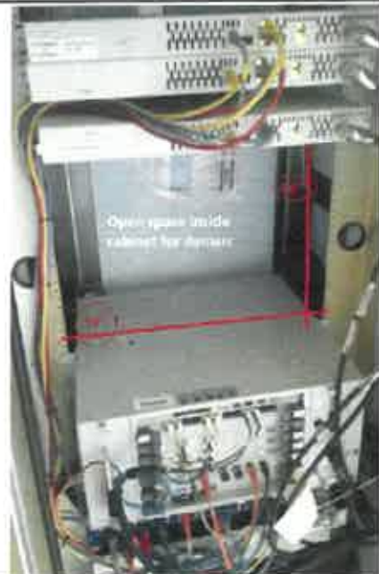
INSIDE MMBTS CABINET
