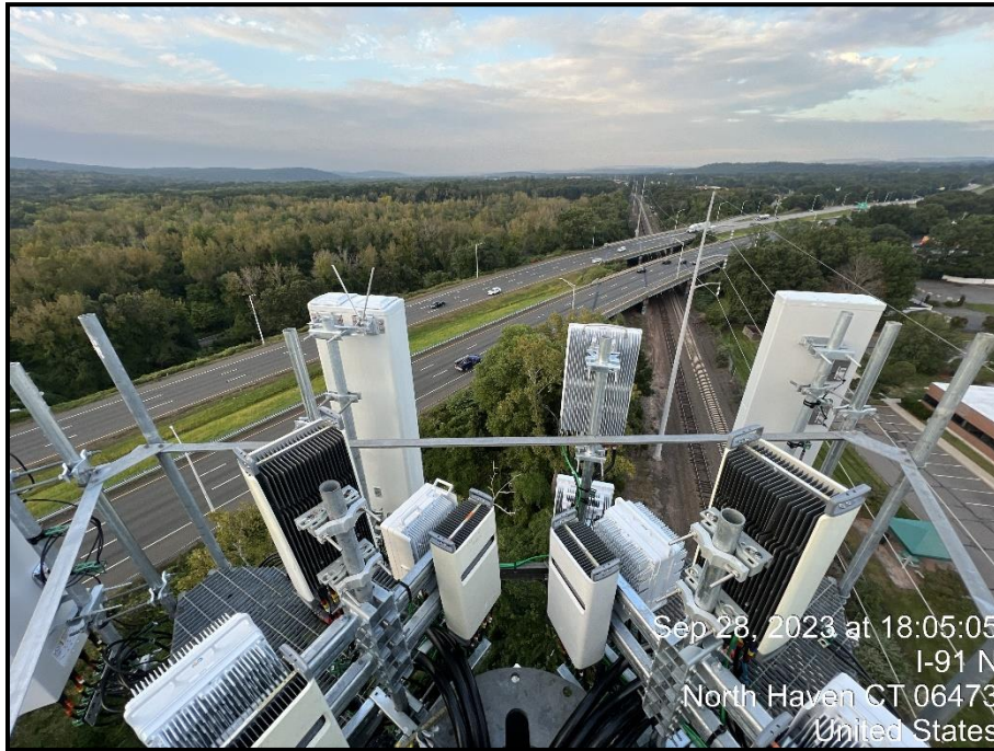
Figure 1: View of installed alpha sector antennas and RRUs on existing mount platform
