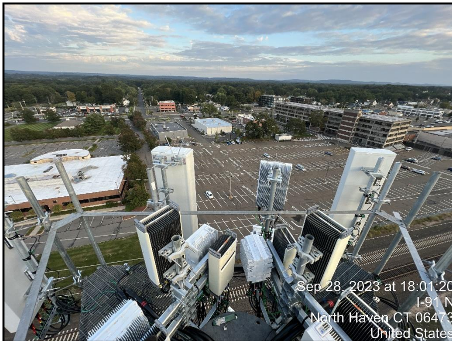
Figure 2: View of installed beta sector antennas and RRUs on existing mount platform
