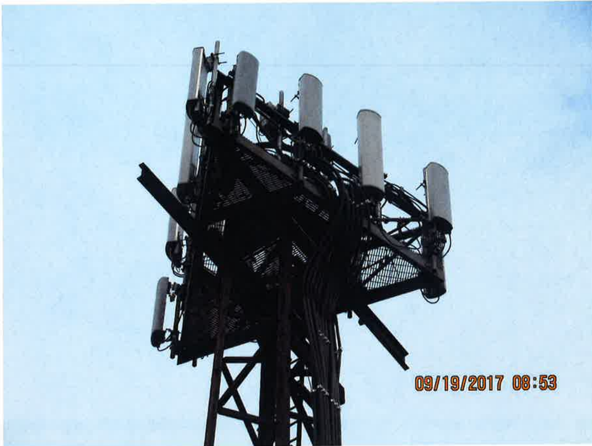
Photo 1: Photo illustrating the Tower with Appurtenances shown.
