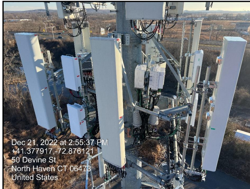
Figure 1: View of installed alpha sector antennas and RRUs on existing mount platform
