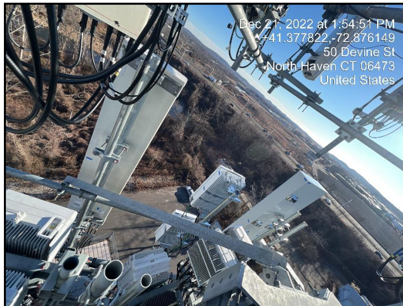
Figure 2: View of installed beta sector antennas and RRUs on existing mount platform
