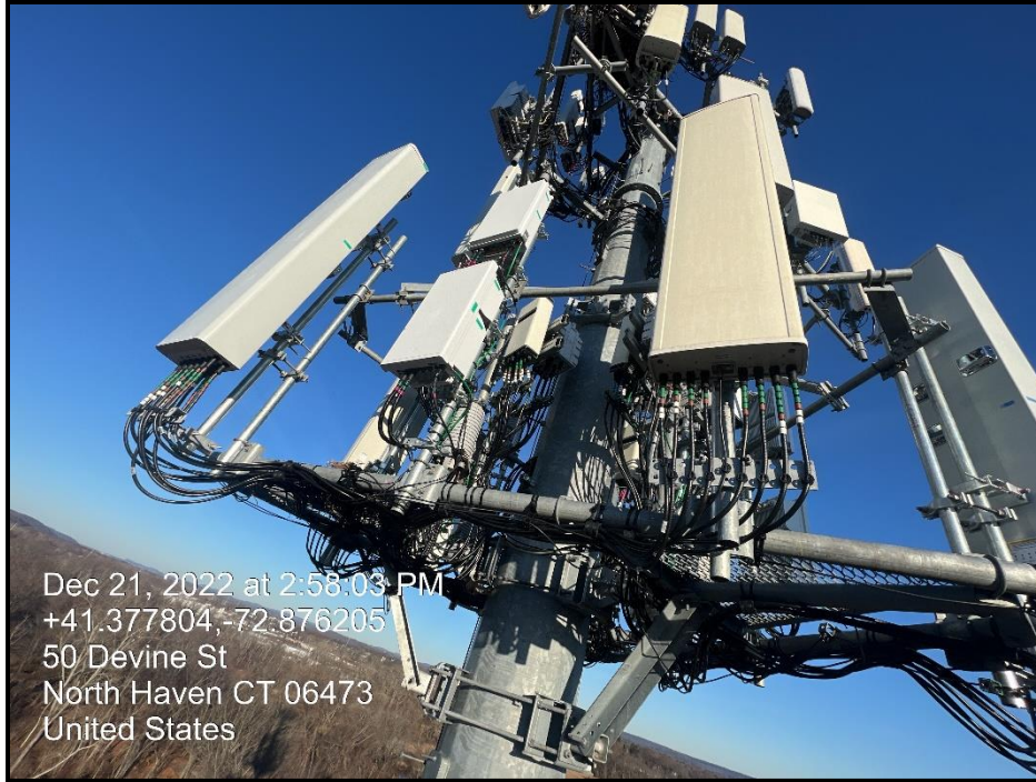
Figure 3: View of installed gamma sector antennas and RRUs on existing mount platform
