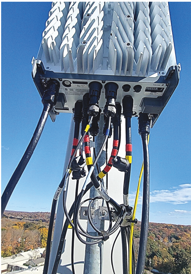
New RRH installed to existing pipe
