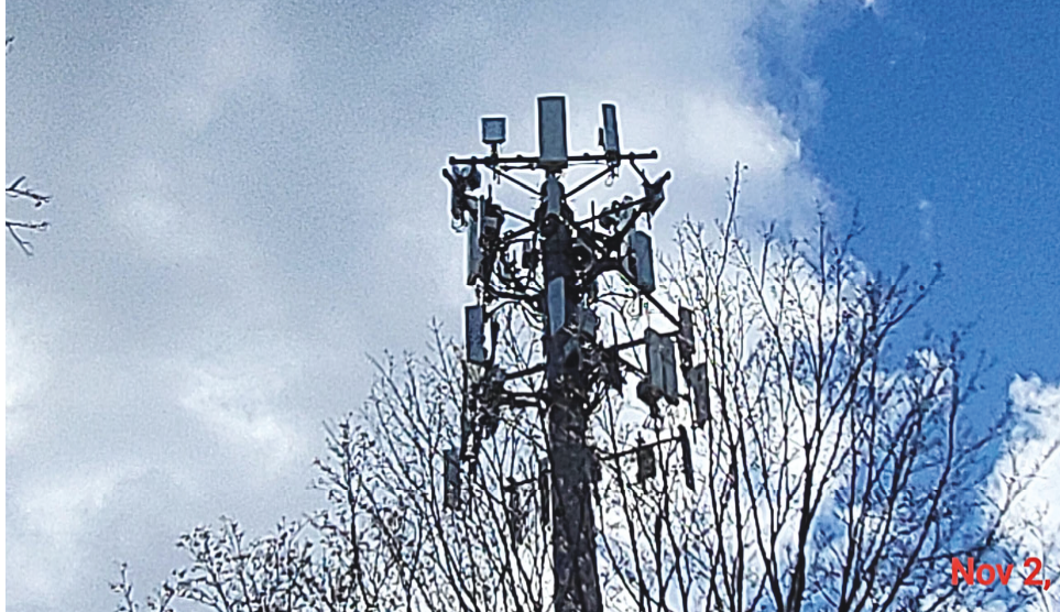
Alpha sector antennas installed on existing sector frame
