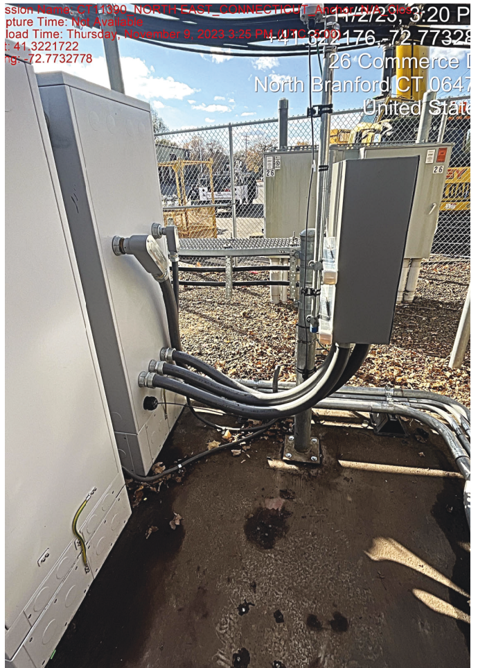
Conduit and ground connections at rear of cabinets
