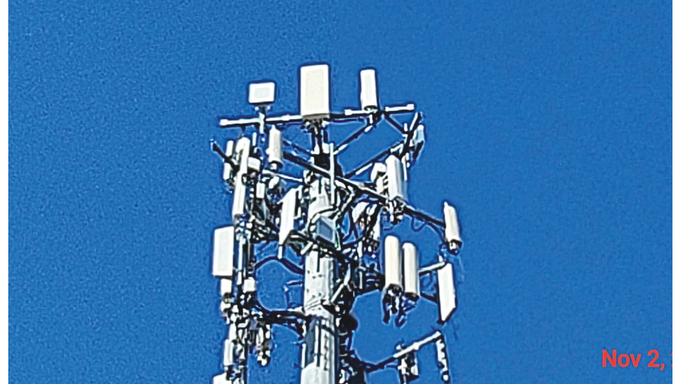
Gamma sector antennas installed on existing sector frame
