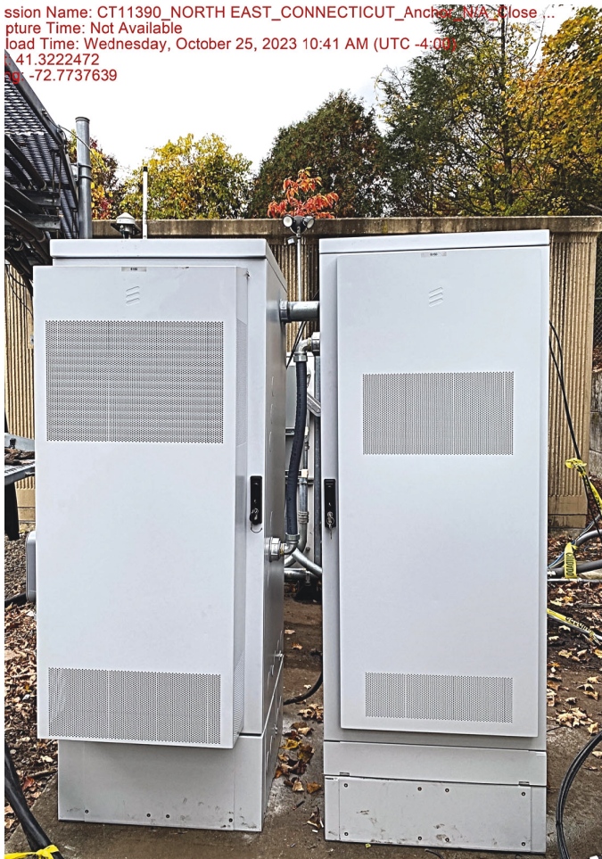
New equipment cabinets installed on concrete pad
