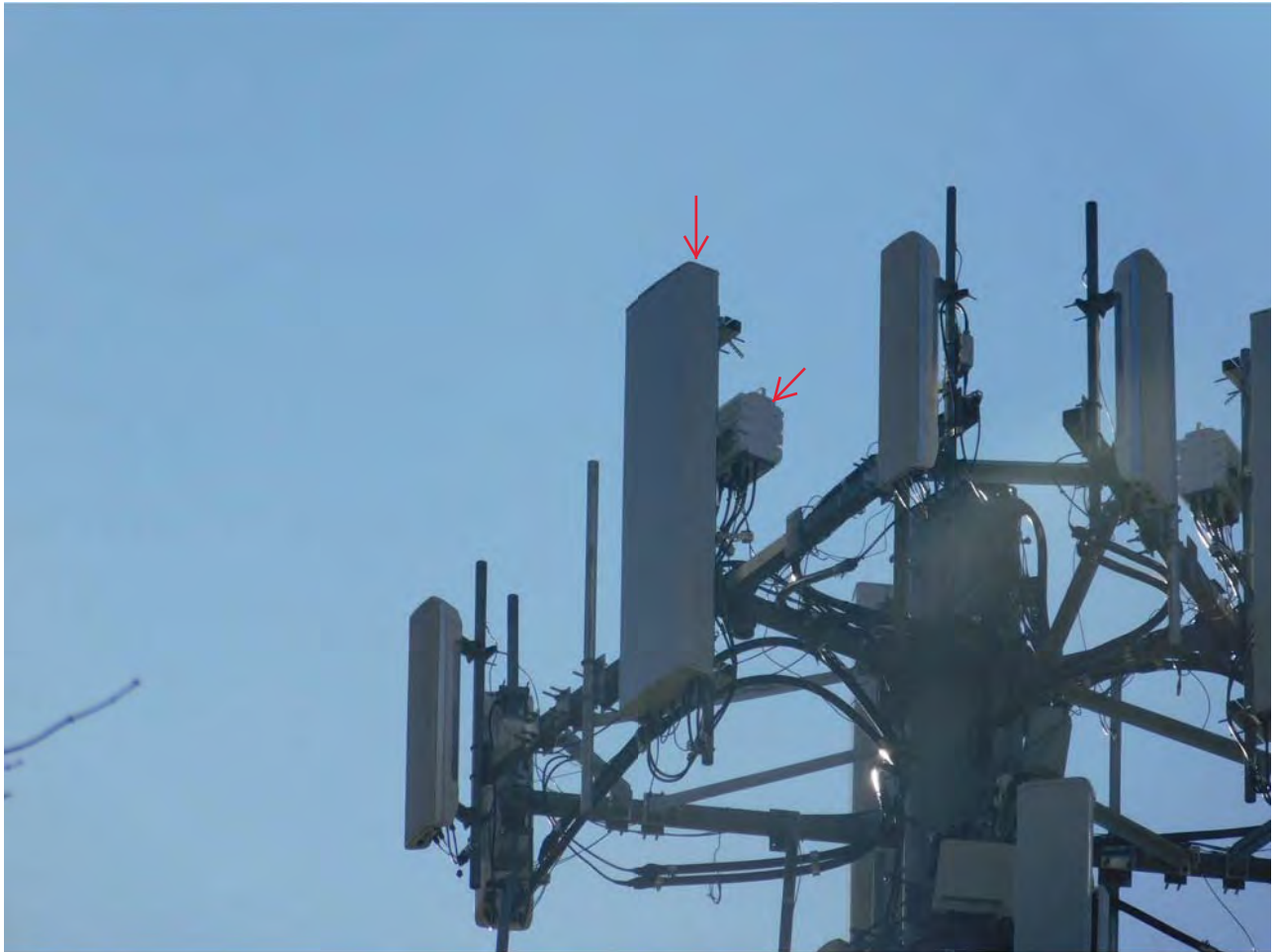
Alpha Sector: (1) New Antenna & (1) New RRH Mounted To The Reinforced Sector Frame
