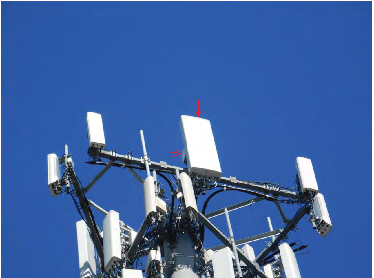
Beta Sector: (1) New Antenna & (1) New RRH Mounted To The Reinforced Sector Frame
