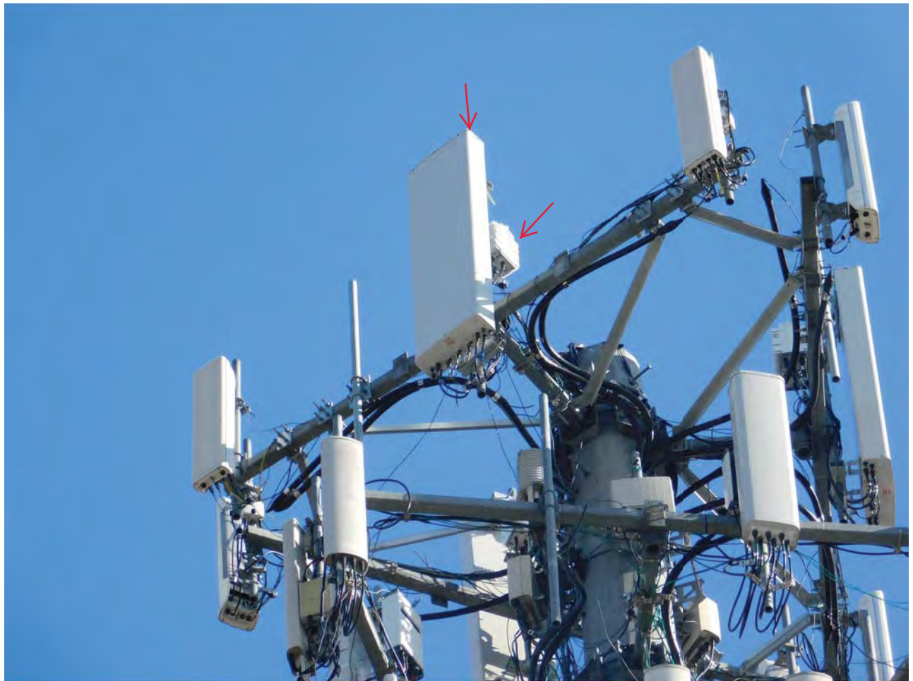
Gamma Sector: (1) New Antenna & (1) New RRH Mounted To The Reinforced Sector Frame
