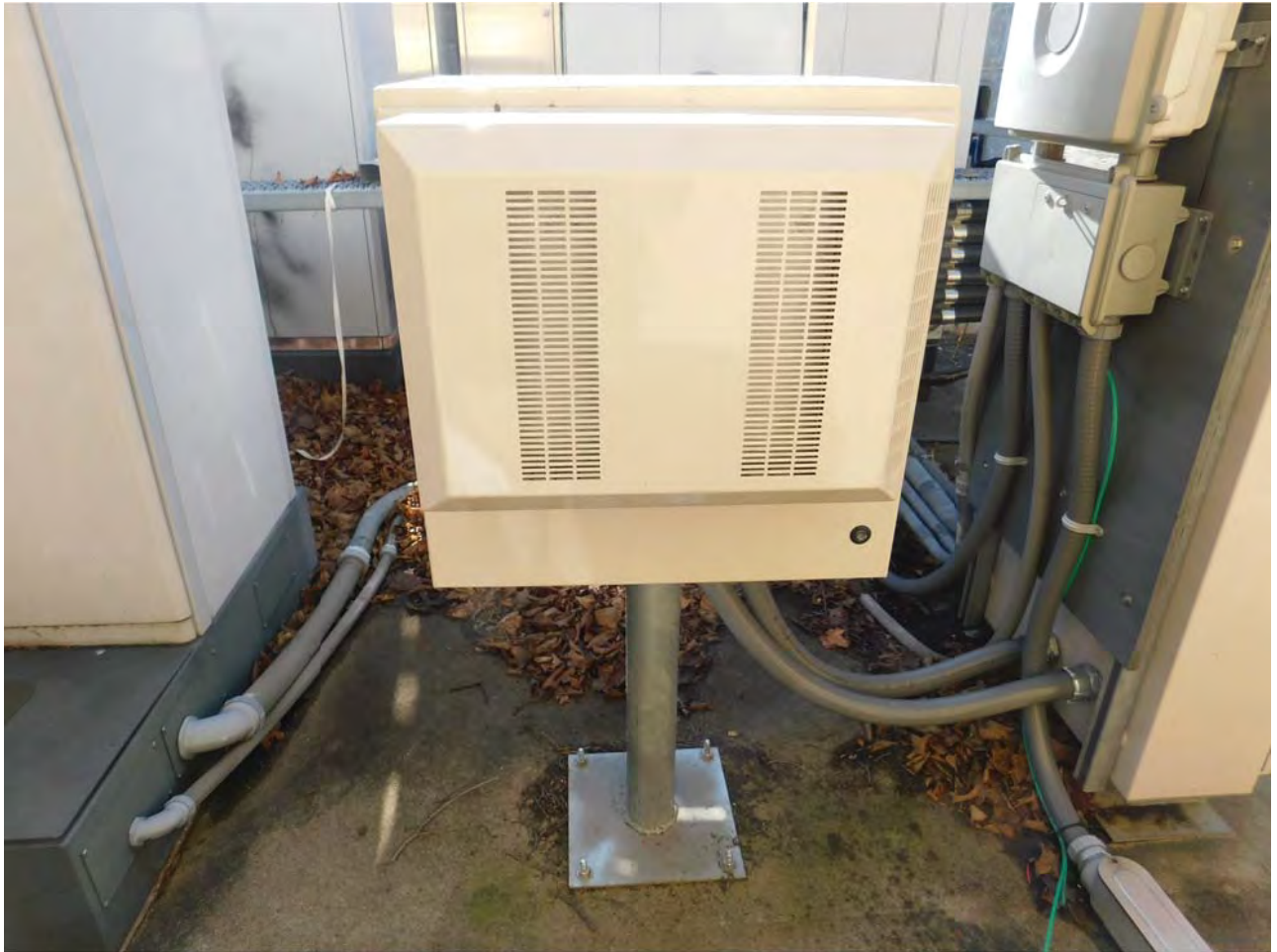
New Purcell Cabinet Mounted To Existing Concrete Pad On A New Mounting Pedestal
