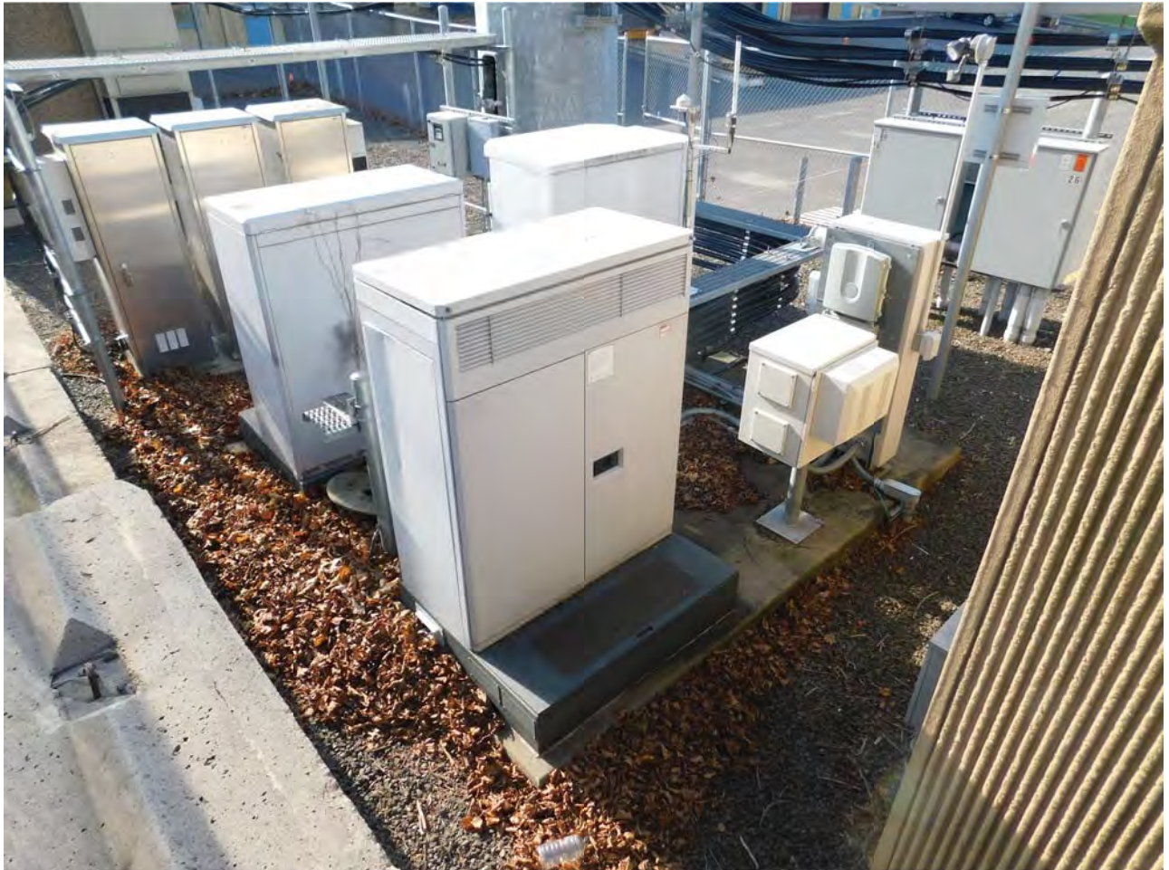
Existing Equipment Cabinets Mounted To Existing Concrete Pad In Existing Compound
