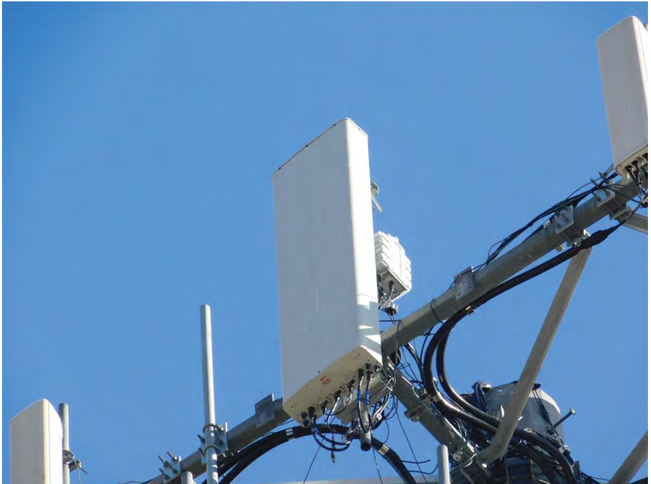
New Antenna & RRH Mounted To The Reinforced Sector Frame (Typical)
