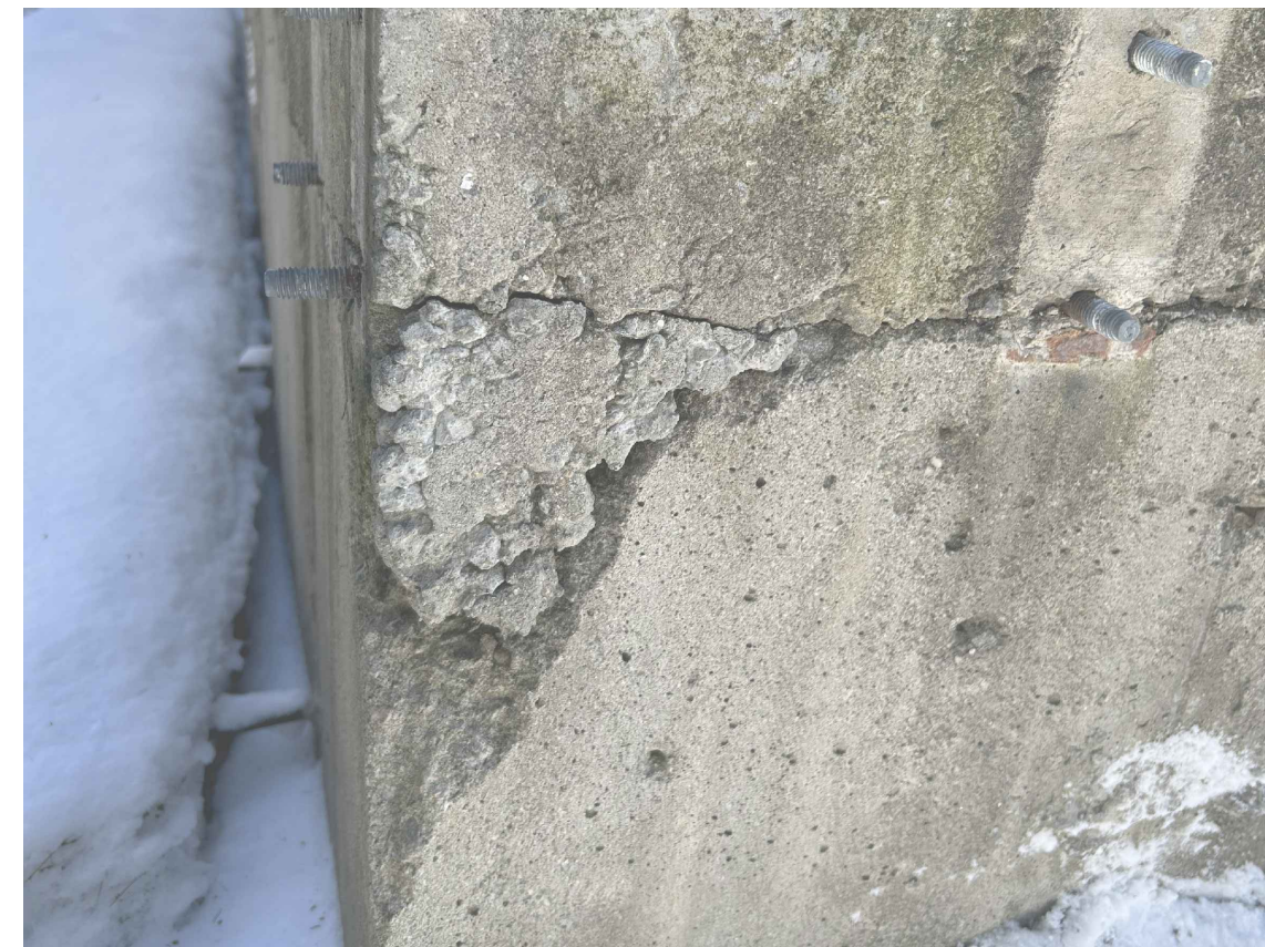
3 BROKEN FOUNDATION CORNER
