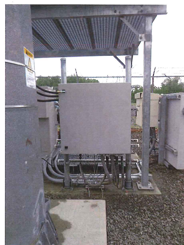
4 EXIST FIBER DISTRIBUTION BOX SCALE: NTS
