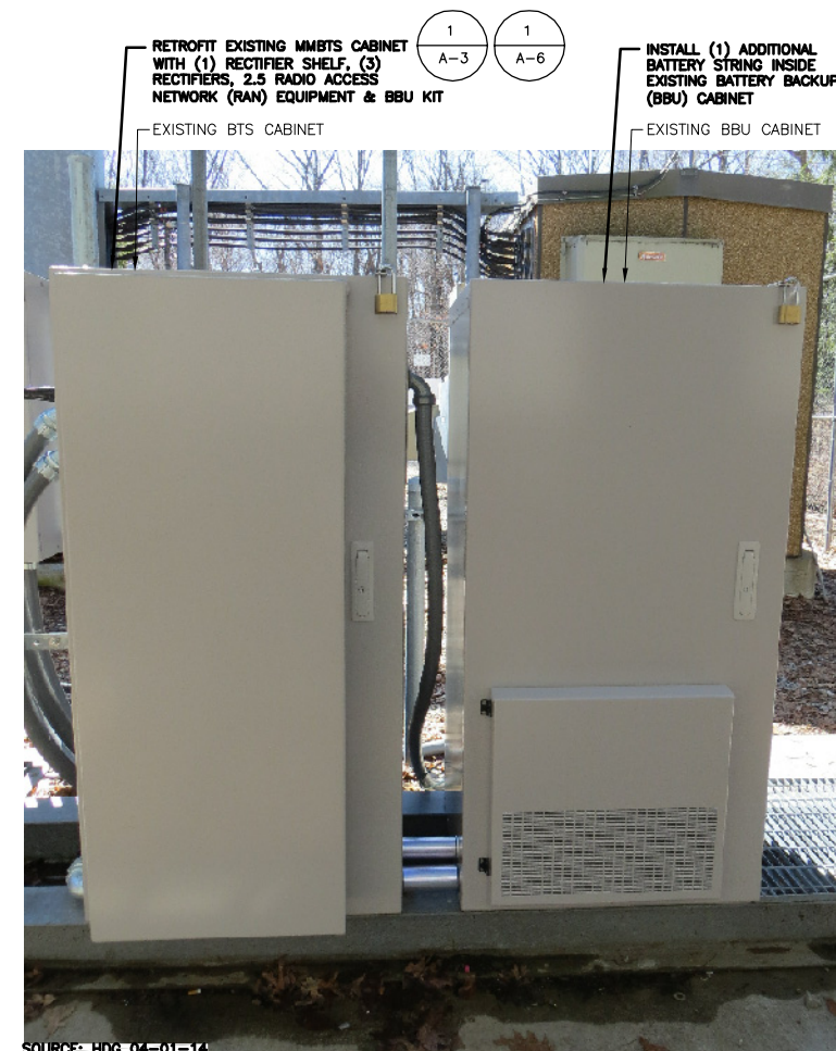
RAN EQUIPMENT PHOTO DETAIL SCALE: N.T.S.
