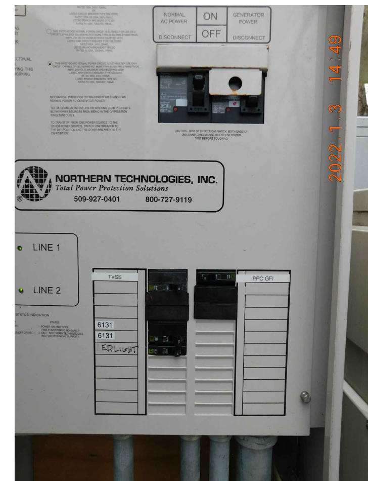
EXISTING POWER PANEL PHOTO SCALE: NOT TO SCALE
