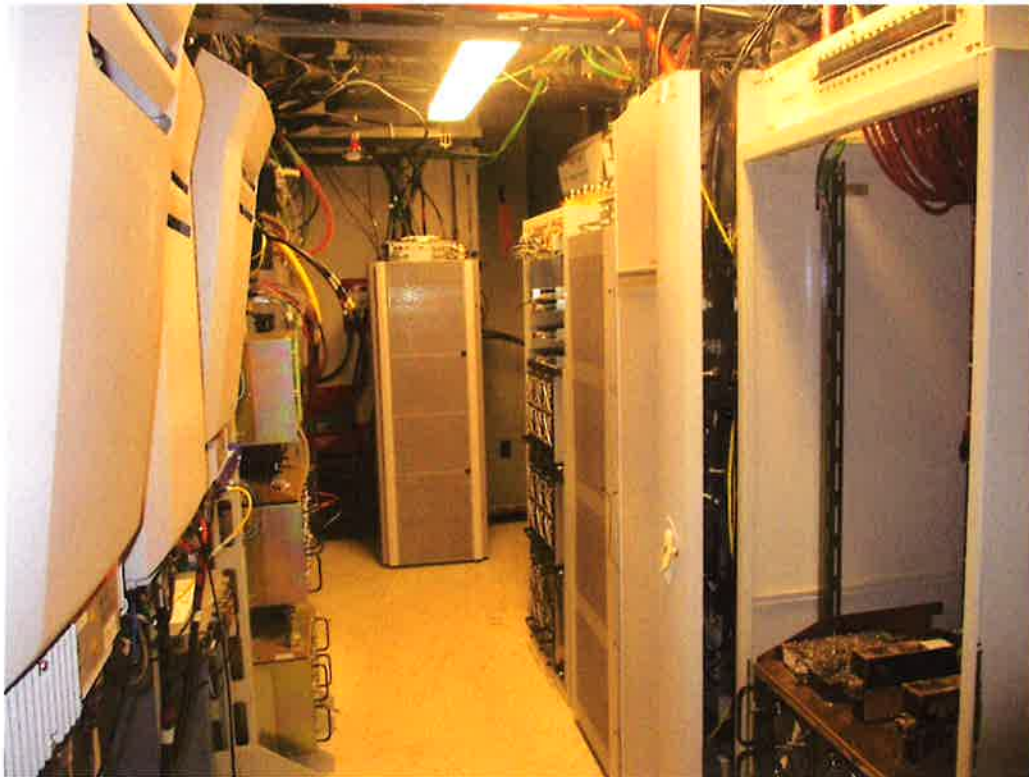
Photo 4: Sample photo illustrating the existing equipment room.
