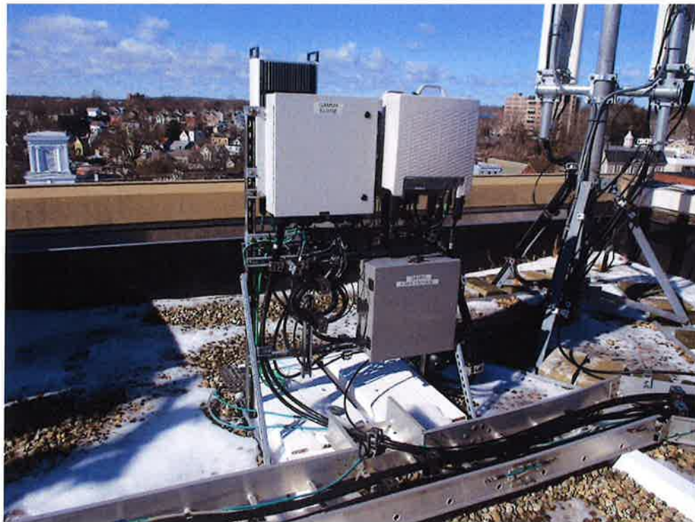
Photo 2: Sample photo illustrating the existing RRH's mounted on the existing Non-penetrating ballast mount.
