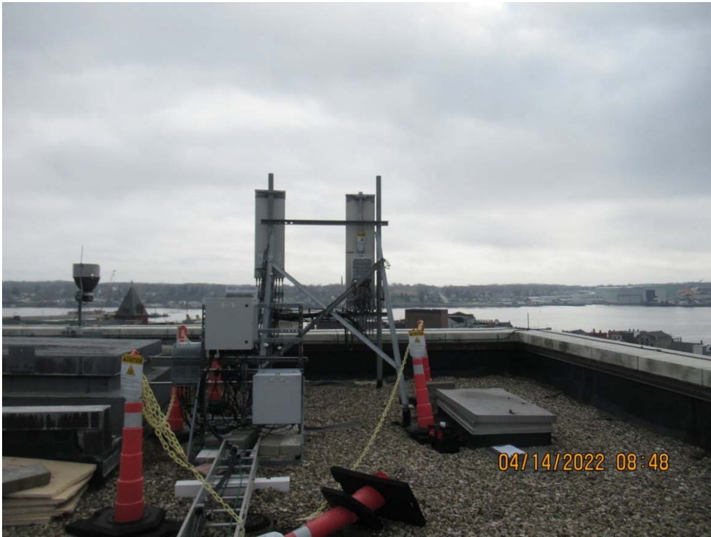
Photo 1: Sample photo illustrating the existing Alpha sector.
