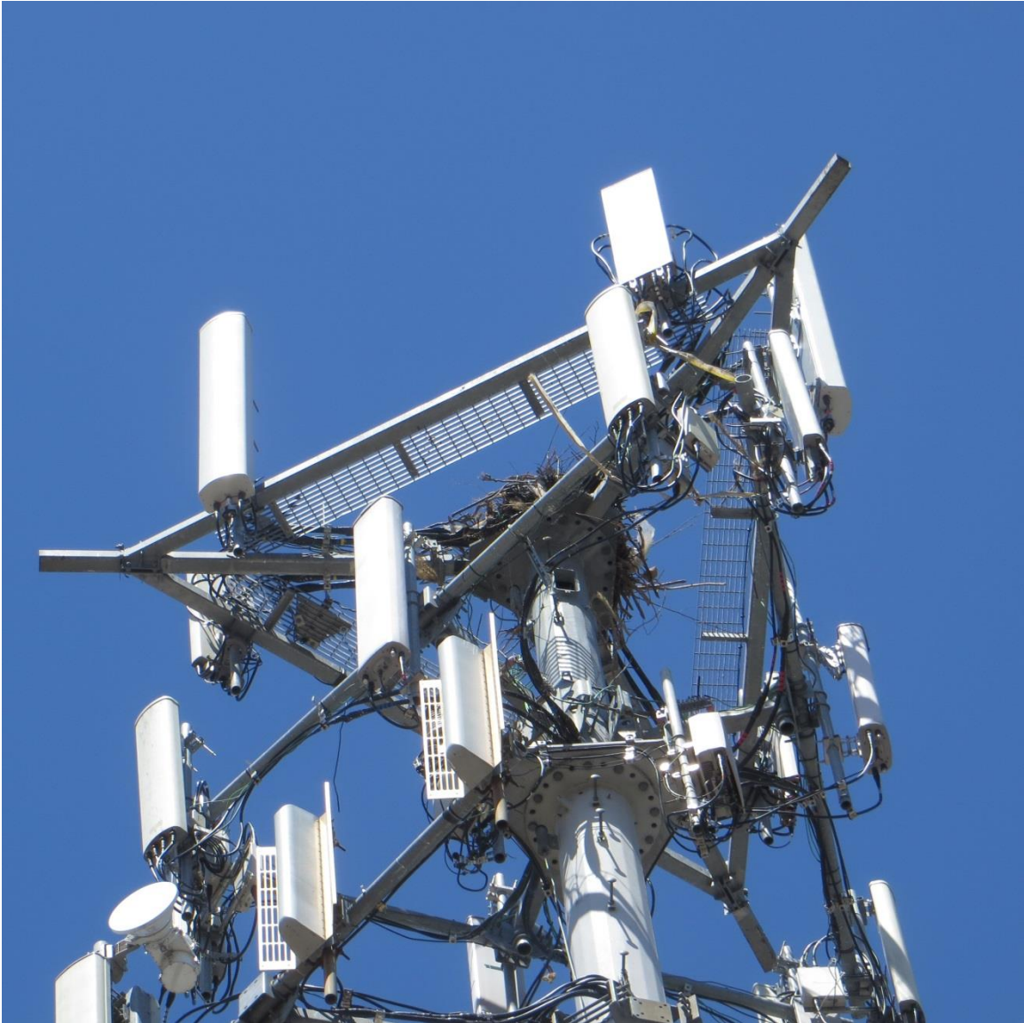
Photo 1: Photo illustrating the Monopole with Appurtenances shown.
