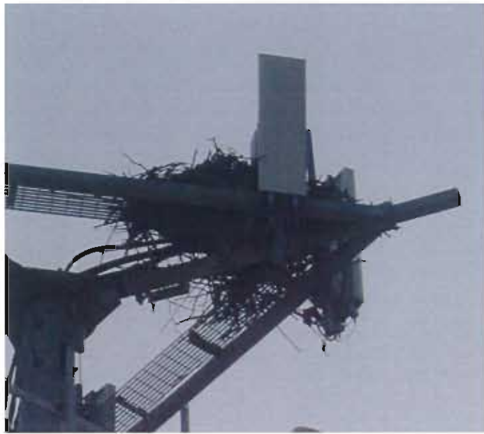
ISSUE #1: LARGE BIRD NEST ON TOP OF TOWER. RECOMMENDATION: REMOVE NEST IF FOUND TO BE UNINHABITED.
