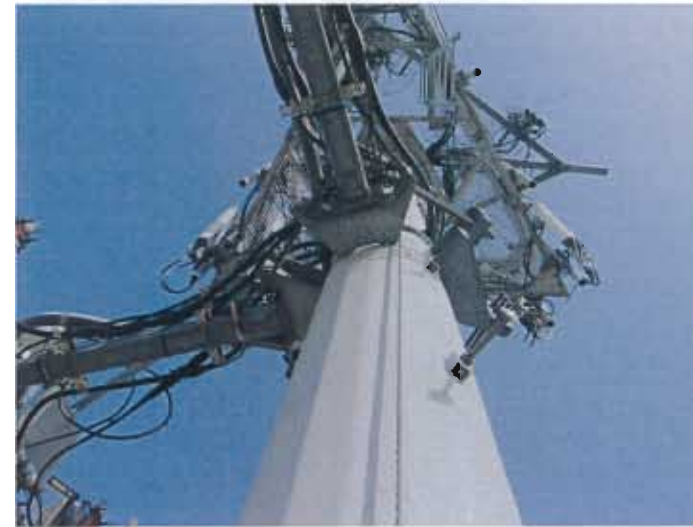
ISSUE #2: SAFETY CLIMB OBSTRUCTED BY MOUNT AT 79' RECOMMENDATION: INSTALL COMPETENT CLIMBER SIGN AT BASE OF TOWER.
