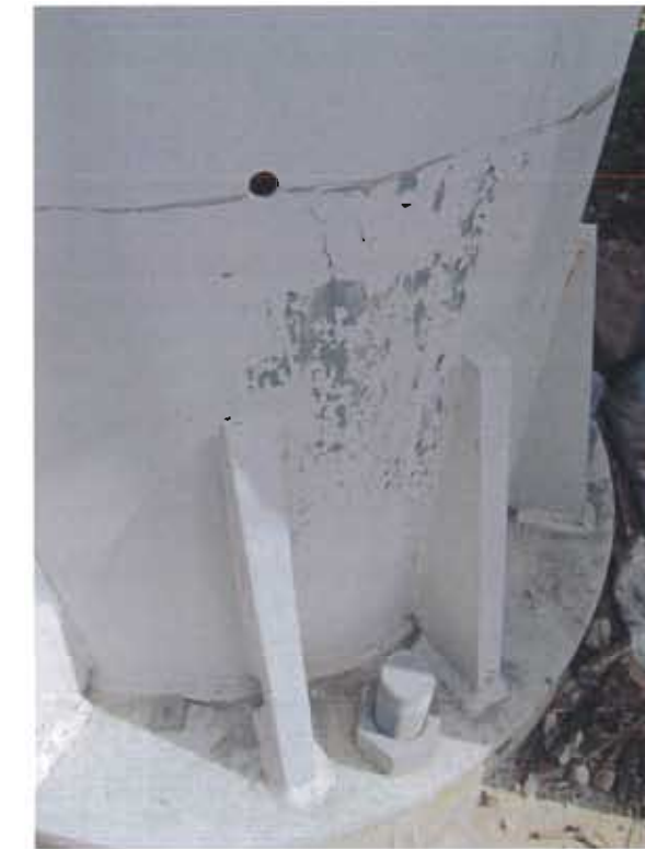
ISSUE #5: PAINT PEELING AROUND BASE OF TOWER. RECOMMENDATION: REMOVE PAINT FROM AFFECTED AREAS USING WIRE BRUSH OR SIMILAR, REPAINT SURFACE WITH MIN. (2) COATS SIMILAR COLOR.
