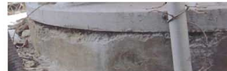
ISSUE #6: GROUT CHIPPING BELOW TOWER BASE PLATE. RECOMMENDATION: REPAIR CHIPS WITH MIN. 4000 PSI NON-SHRINK GROUT & MONITOR GROUT FOR FURTHER CRACKING.
