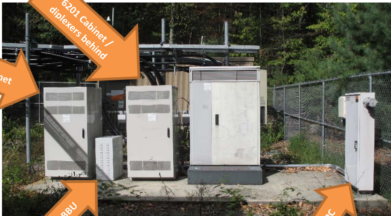
T-Mobile Equipment Area
