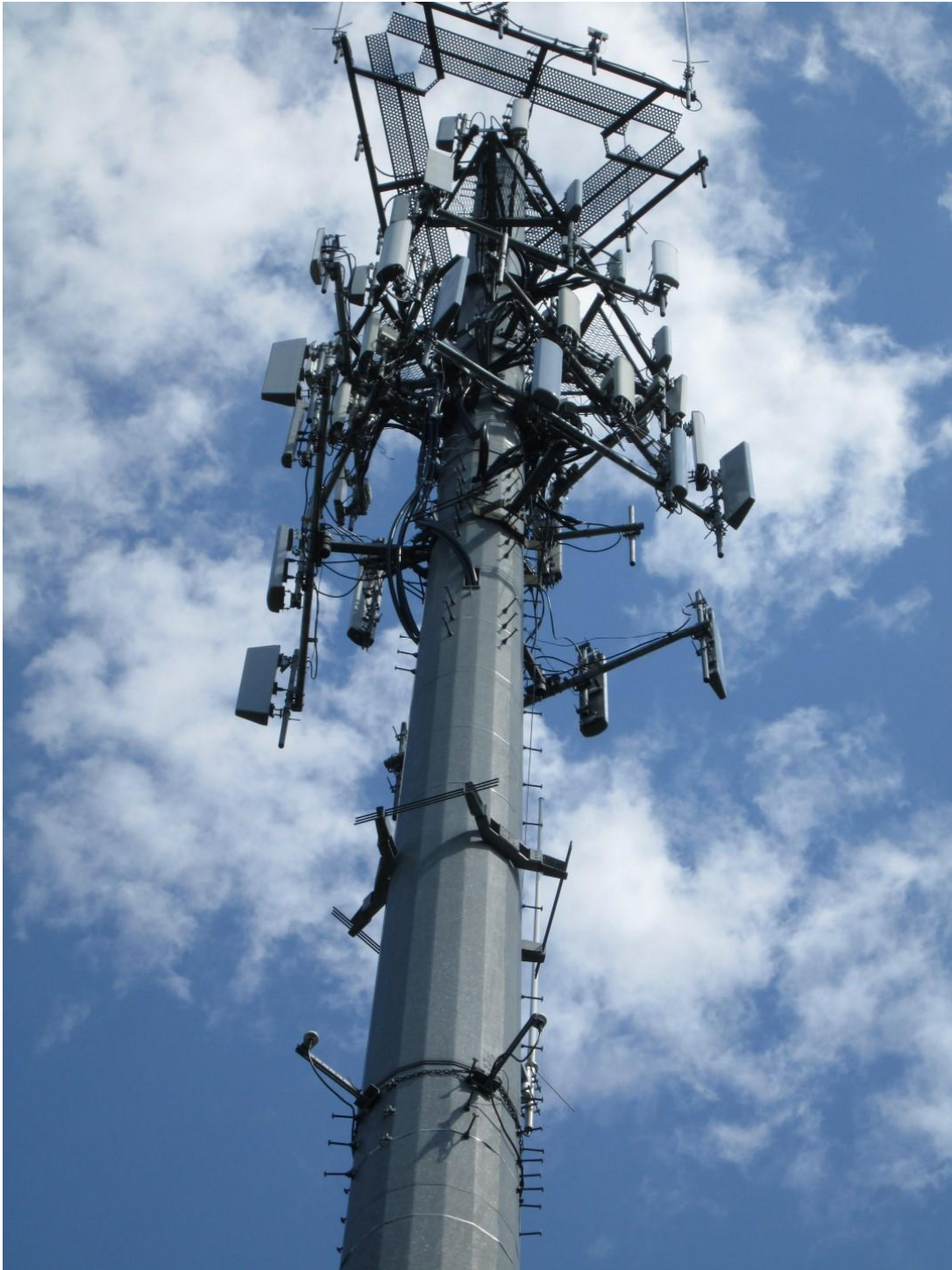
Photo showing existing antennas on upper tower.
