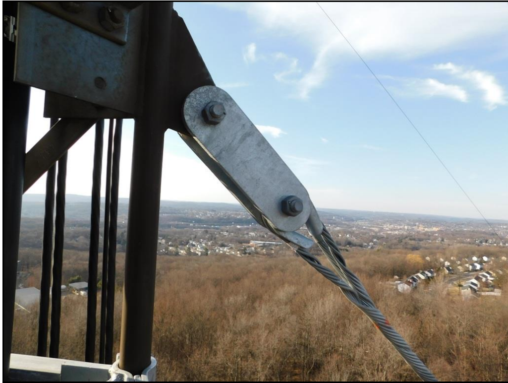
Photo 2A – New guy wire and hardware at the tower end of the wire
