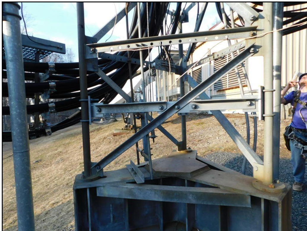
Photo 14 - Existing sub-bracing from 4' to 40' (9 bays) was removed and replaced with new sub-bracing
