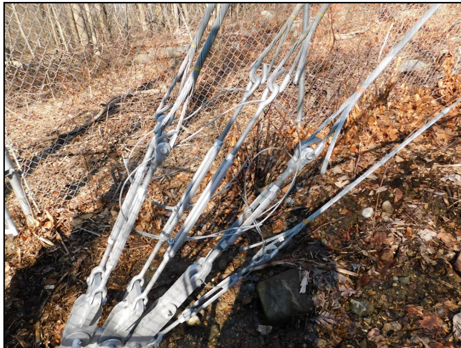
Photo 2 – Another view of new, higher capacity guy wires, levels 1 and 2
