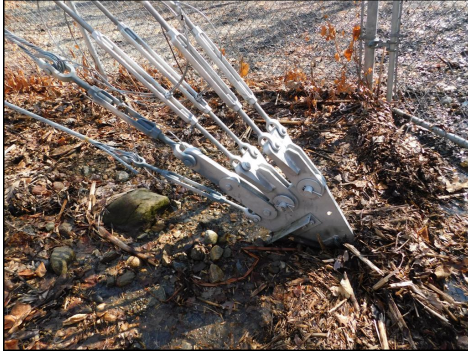
Photo 1 – Replaced existing guy wires at levels 1 and 2 with new, higher capacity guy wires
