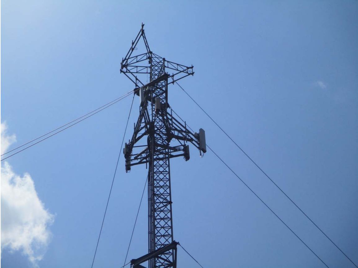
Photo 1: Photo illustrating the Tower with Appurtenances shown.
