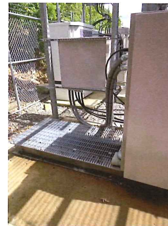
4 EXIST FIBER DISTRIBUTION BOX SCALE: NTS
