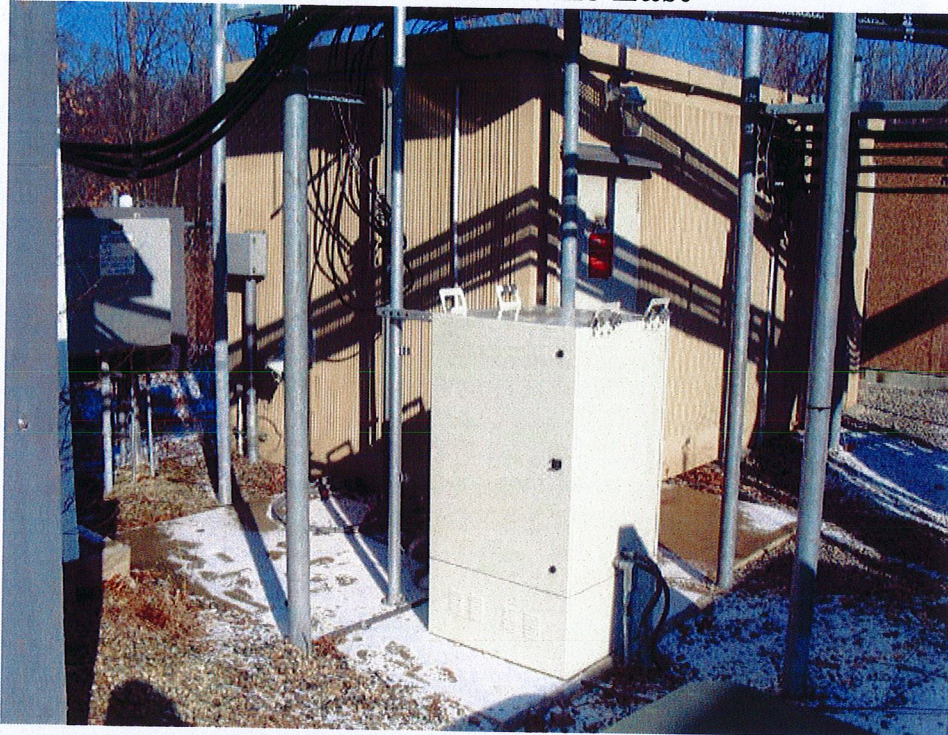
AT&T Base station before removal
