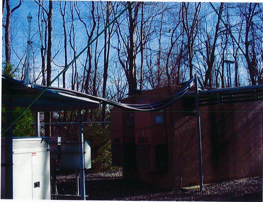
AT&T Base station equipment to be removed
