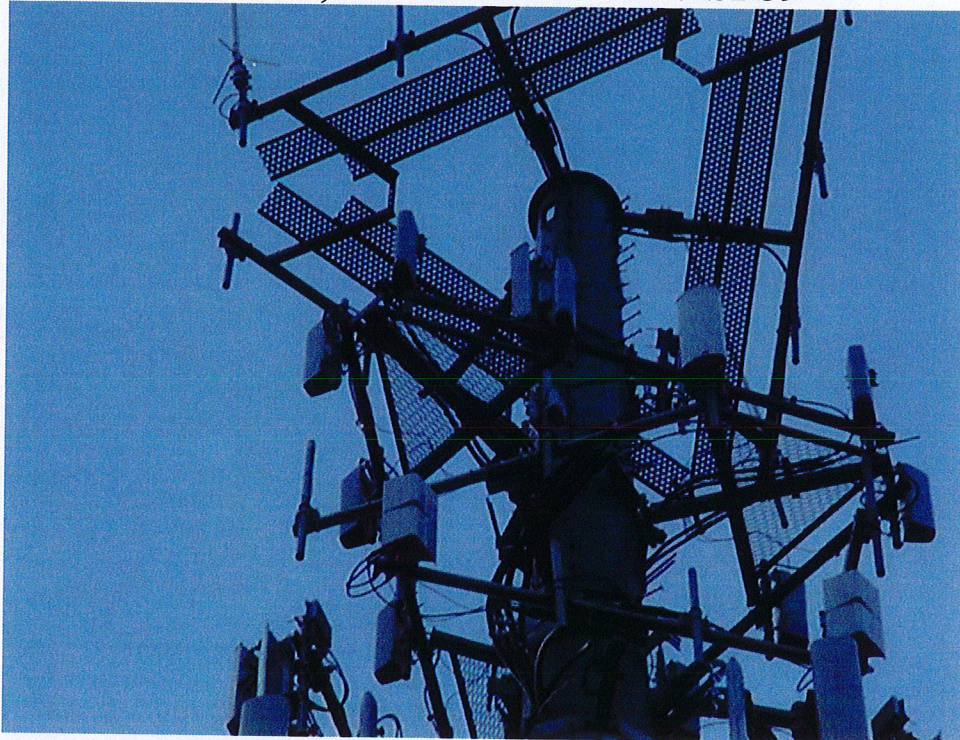
AT&T Allgon panels before removal
