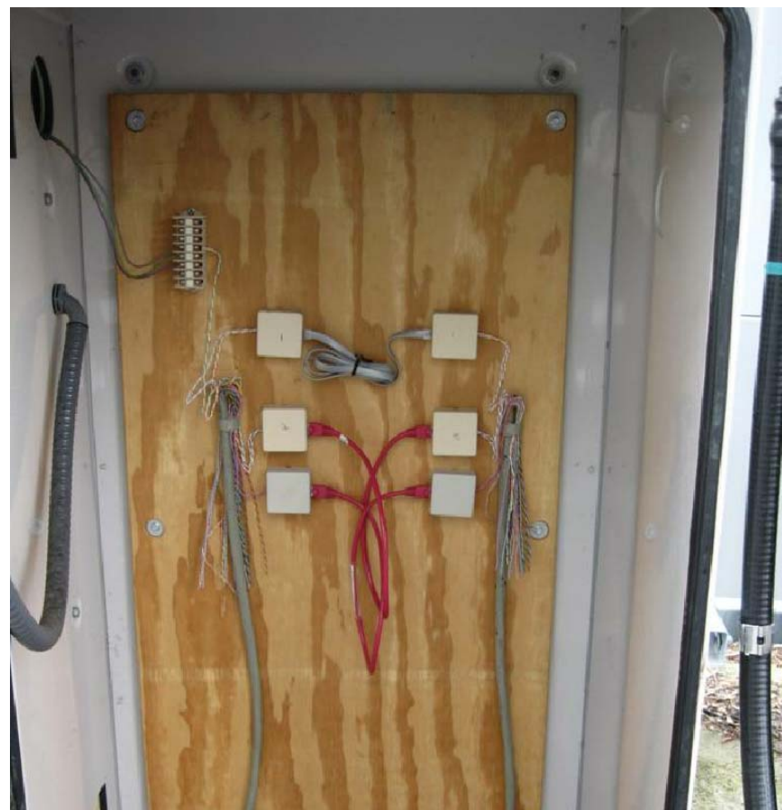
4 EXISTING TELCO CABINET
