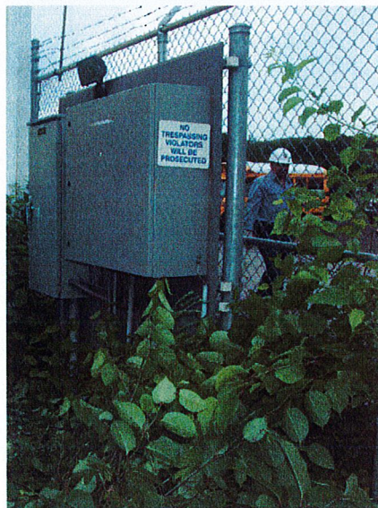
AT&T ELECTRICAL & TELEPHONE EQUIPMENT TO BE REMOVED
