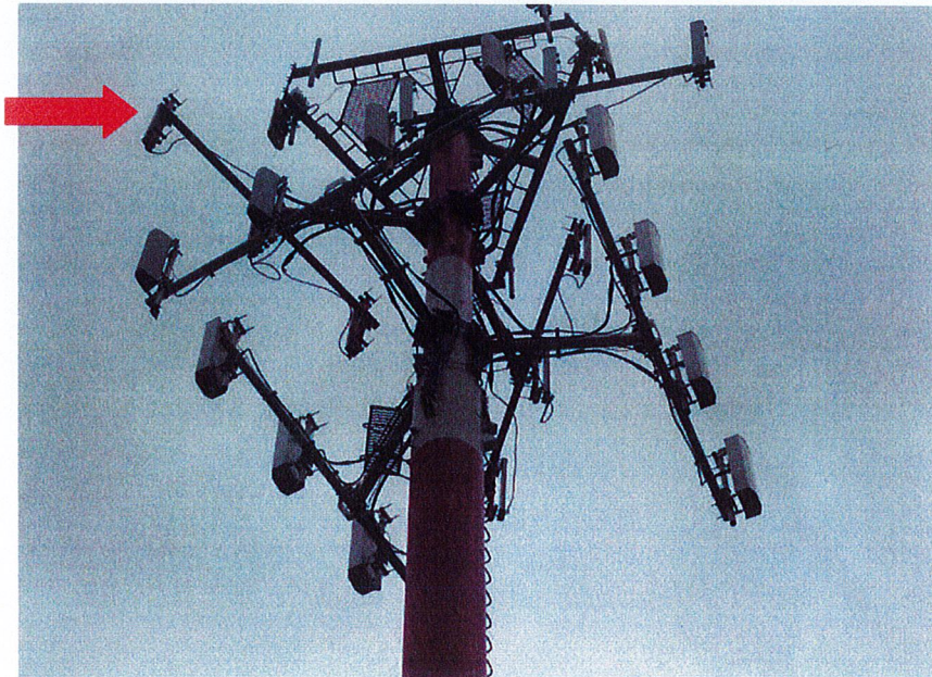
AT&T ARRAY TO BE REMOVED, SHOWN AT 95' (Center Position)
