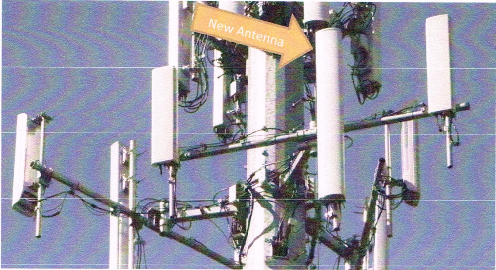
Typical sector showing three new panel antenna (center).
