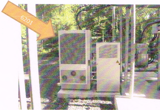
Existing T-Mobile equipment area
