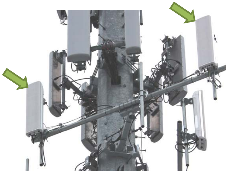
Typical sector showing new panel antennas on new sector frame
