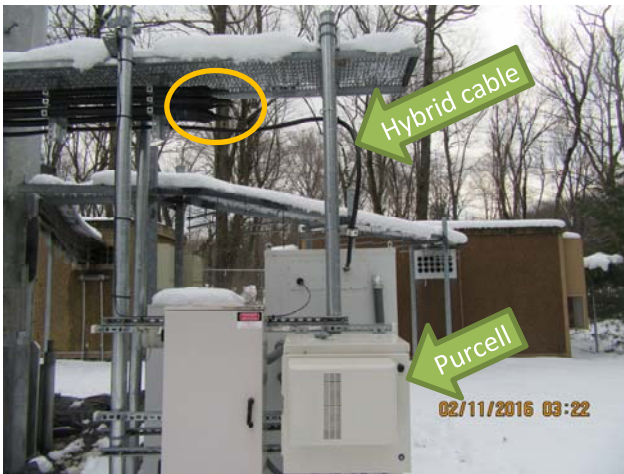
Capped and wrapped existing coaxial cables (circled), new hybrid cable, and Purcell cabinet
