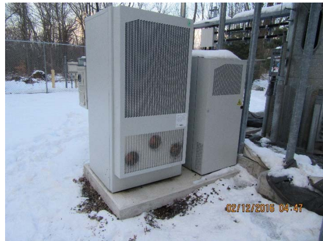
New 6201 cabinet within Delta enclosure (left) and 6101 cabinet (right) on concrete pad
