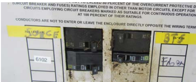
PPC breaker panel with new 60 amp breaker for 6201 cabinet (bottom left) and 20 amp breaker for Purcell cabinet (lower right)
