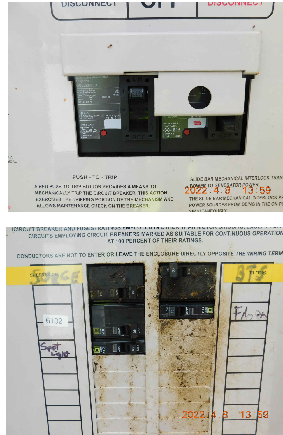
EXISTING POWER PANEL PHOTOS 1 SCALE: NOT TO SCALE
