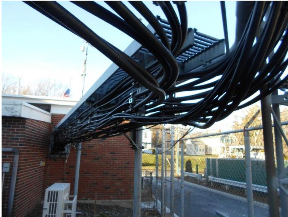
Photo of existing feed lines and ice bridge.
