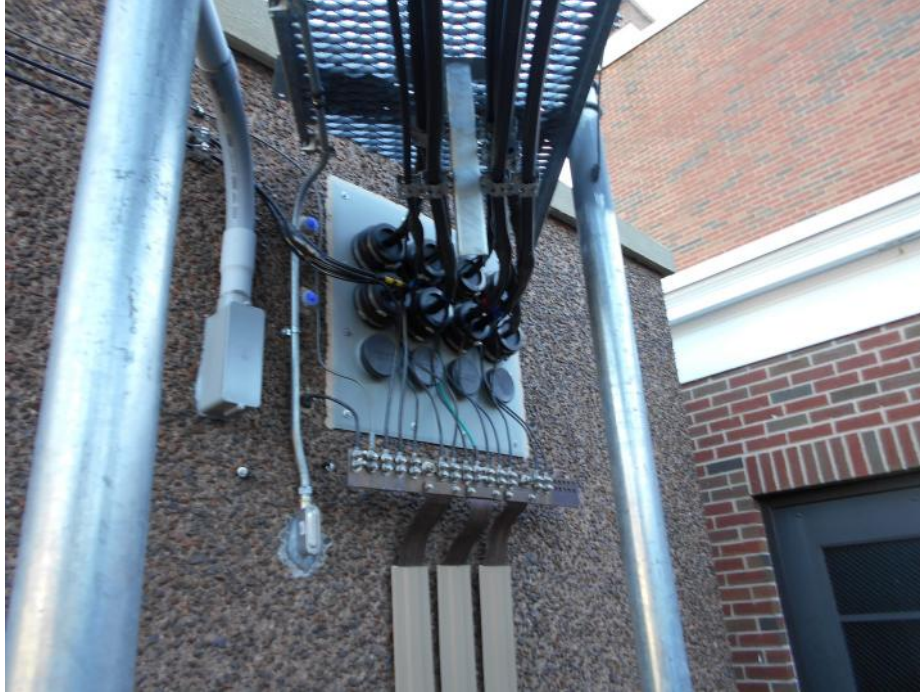
Photo of existing hatch plates and ground bar at shelter.
