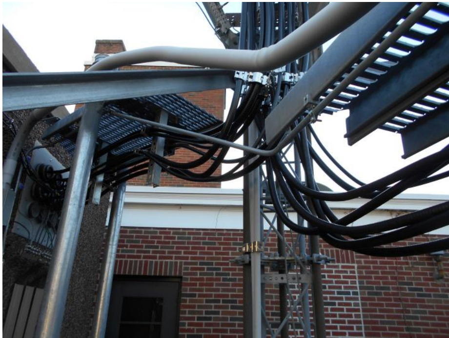
Photo of existing ice bridge and feed lines at tower.
