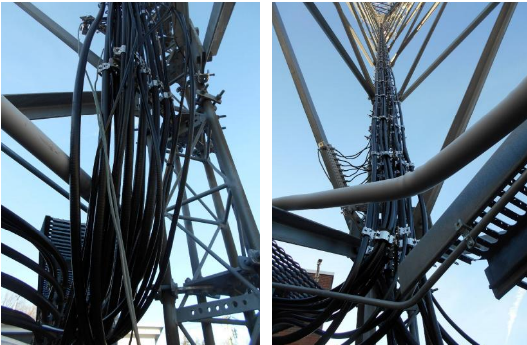
Photos of existing feed lines at tower.
