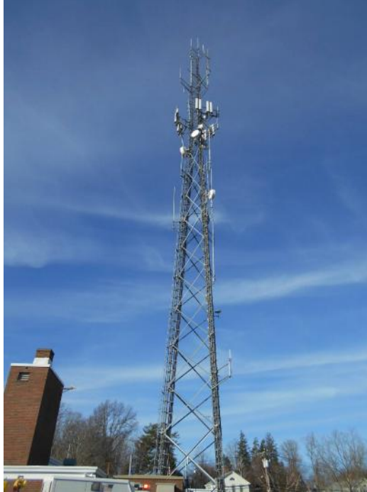
Overview photo of the 180' self-supporting tower located in Middletown, Connecticut.
