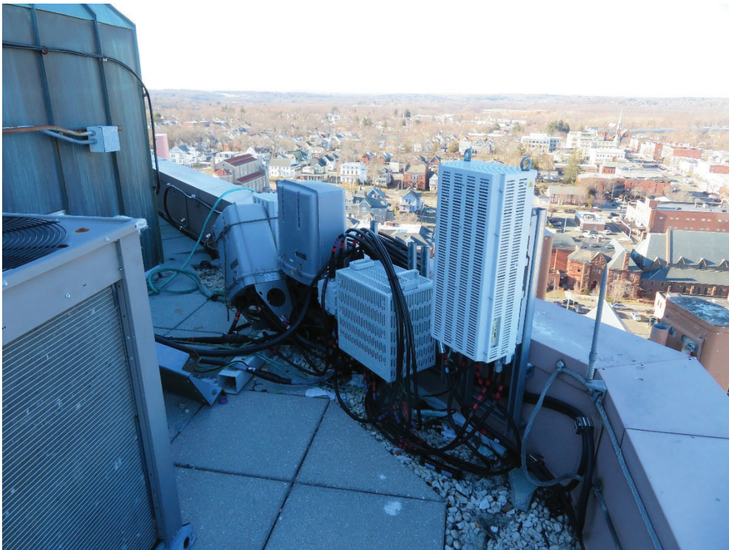
Photo 4: Sample photo illustrating the existing equipment.
