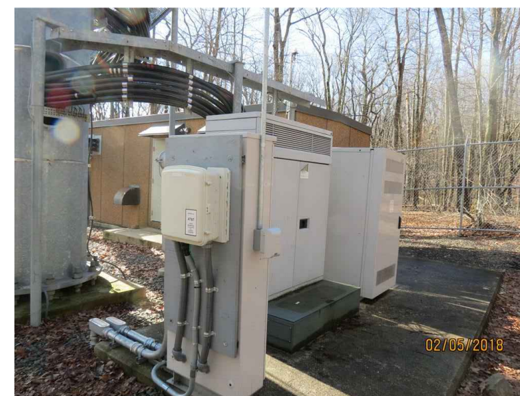
4 EXISTING GROUND EQUIPMENT LAYOUT (LOOKING SOUTH)
