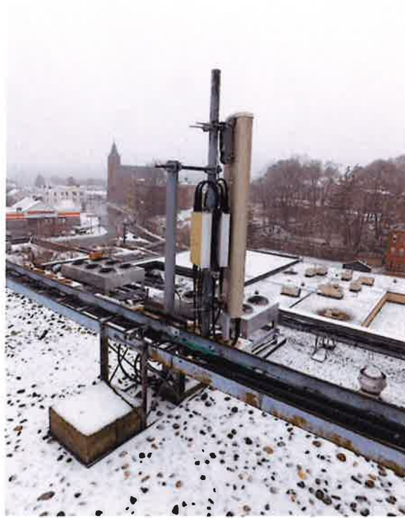
Photo 1: Sample photo illustrating the existing antennas and mounts
