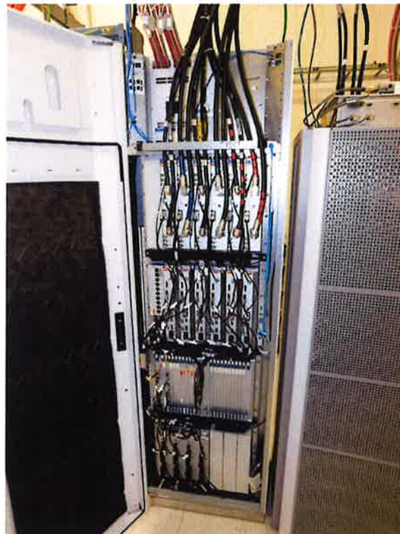
Photo 4: Sample photo illustrating the existing equipment cabinets.
