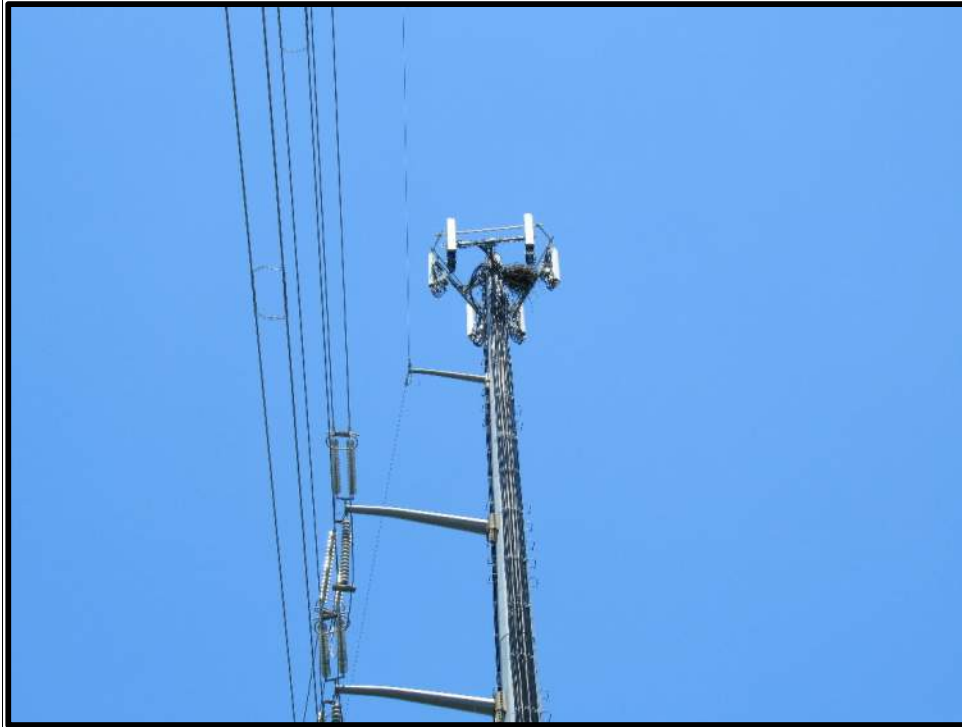
Figure 1: Overview of installed antennas.
