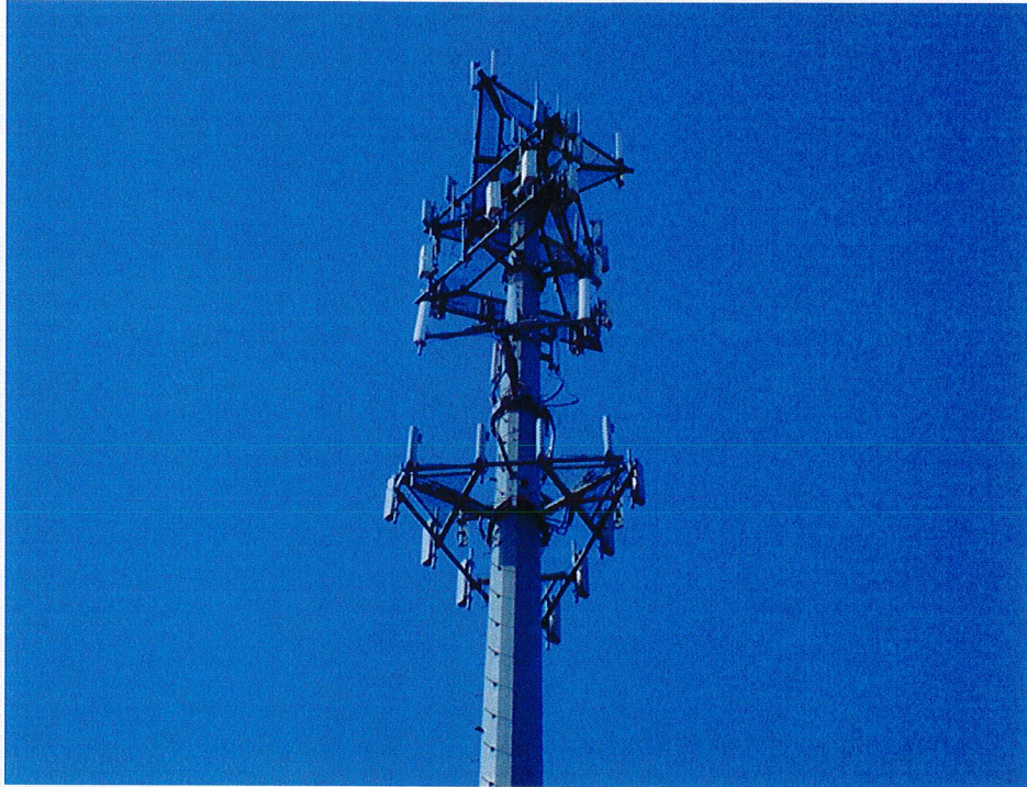
AT&T Allgon 7250.03 antenna before removal (2 nd from top)
