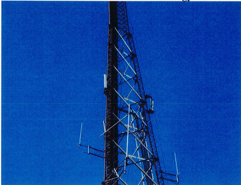
AT&T Allgon 7250.03 antennas before removal
