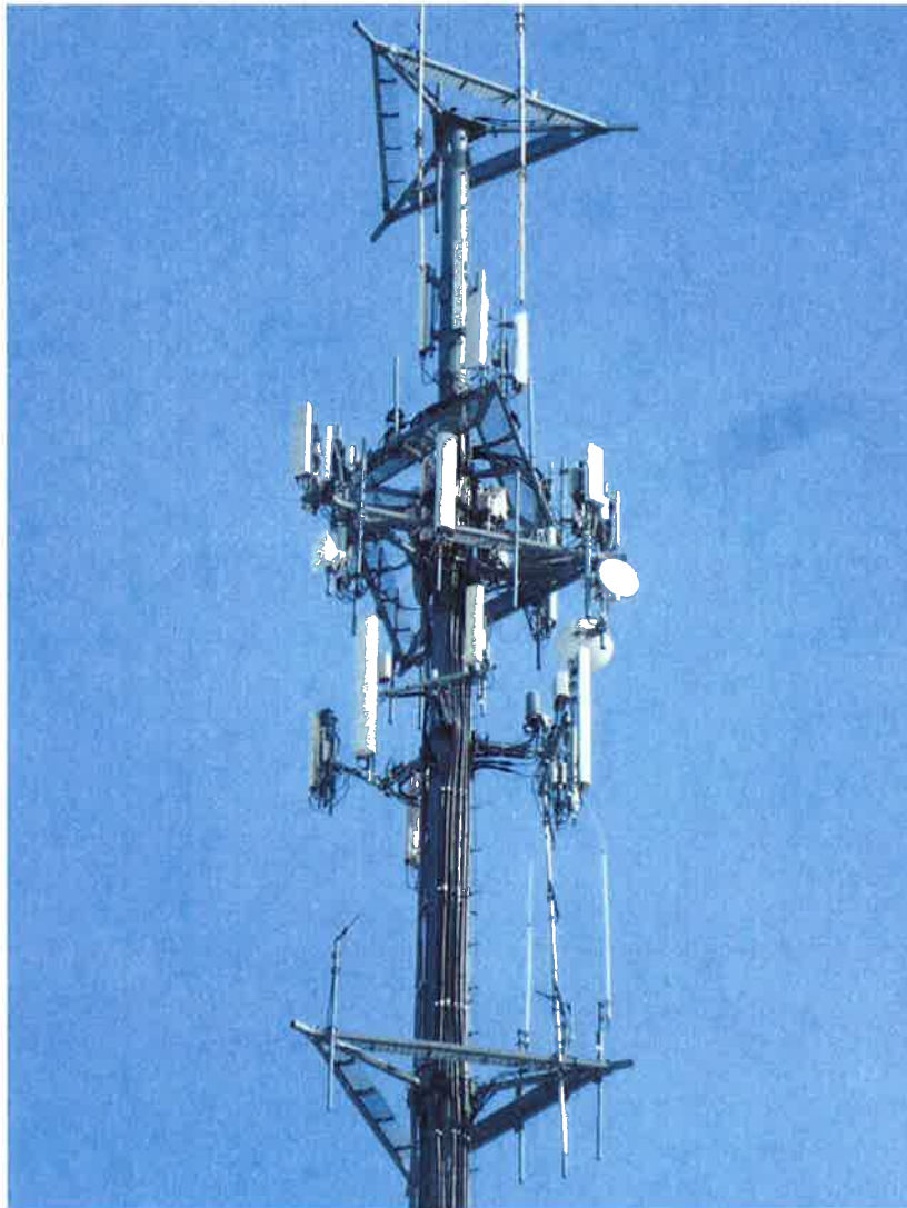
Photo 1: Photo illustrating the Monopole with Appurtenances shown.
