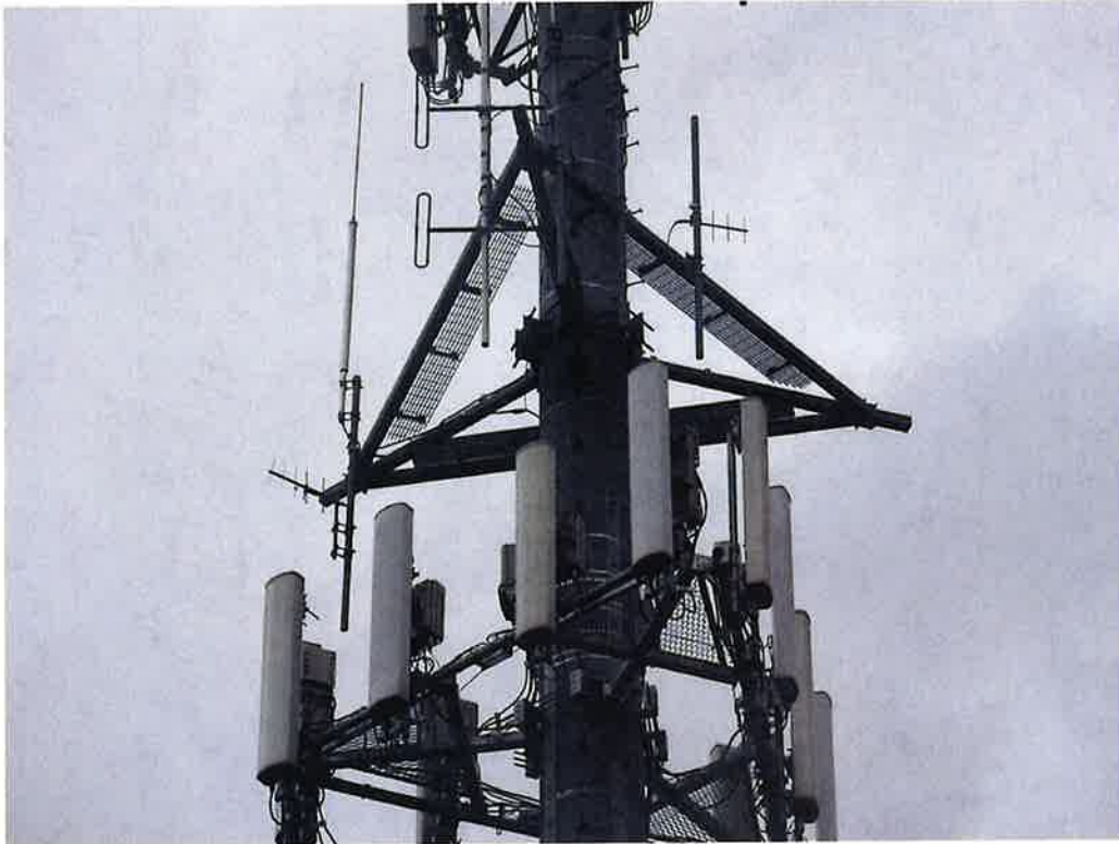
Photo 1: Photo illustrating the Monopole with Appurtenances shown.
