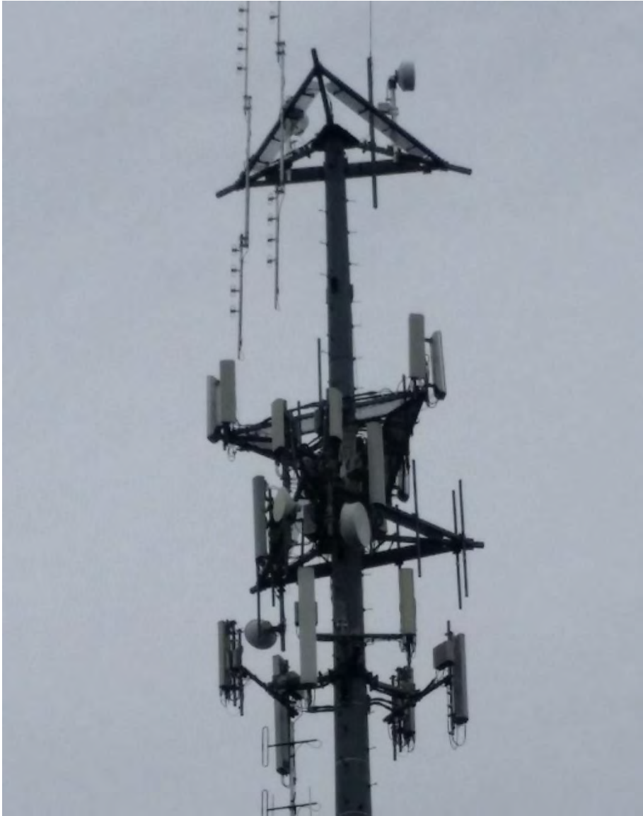
Photo 1: Photo illustrating the Monopole with Appurtenances shown.
