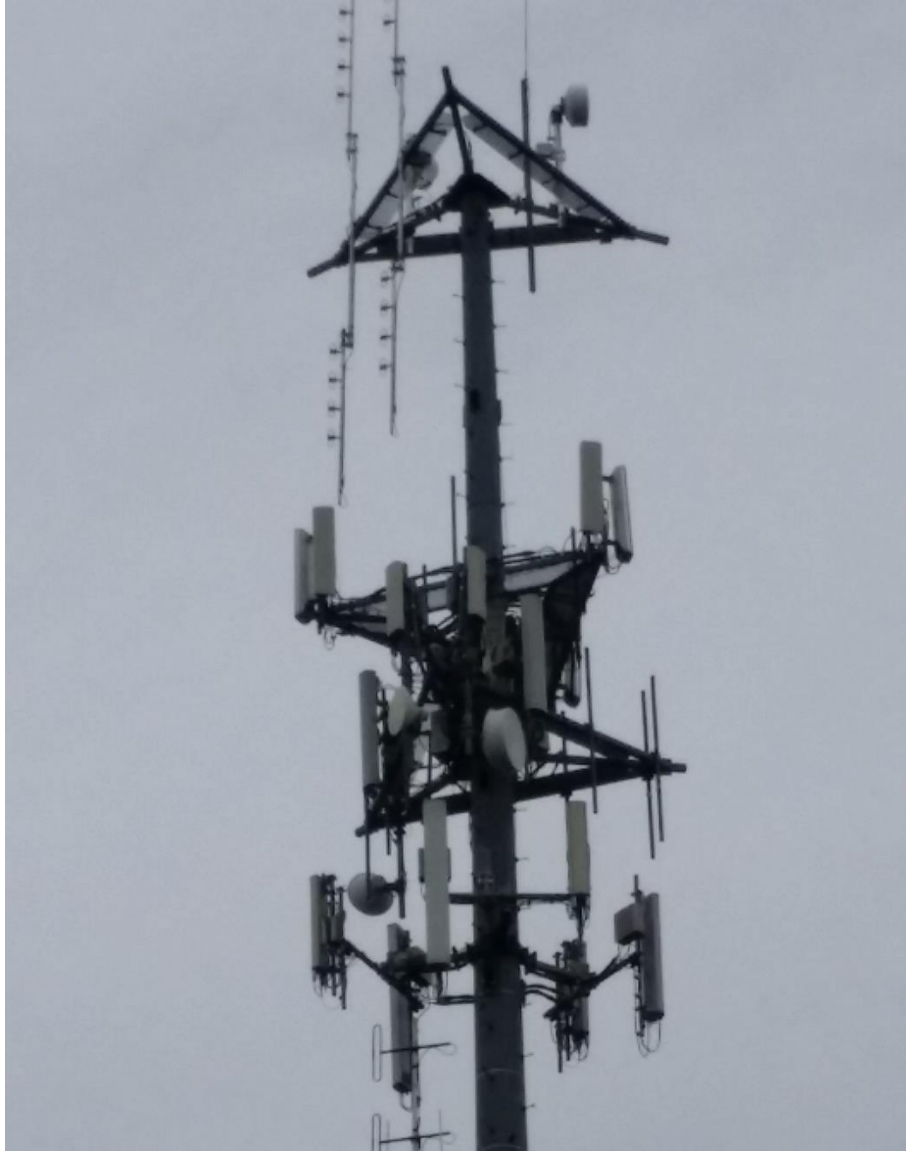
Photo 1: Photo illustrating the Monopole with Appurtenances shown.
