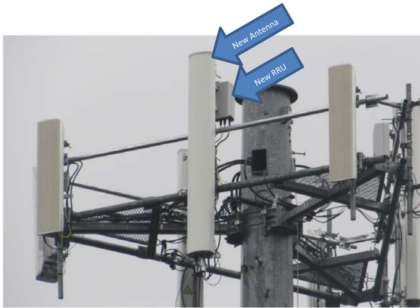
T-Mobile antenna array.
