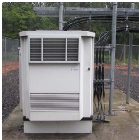
3106 cabinet with 6131 upgrade.
