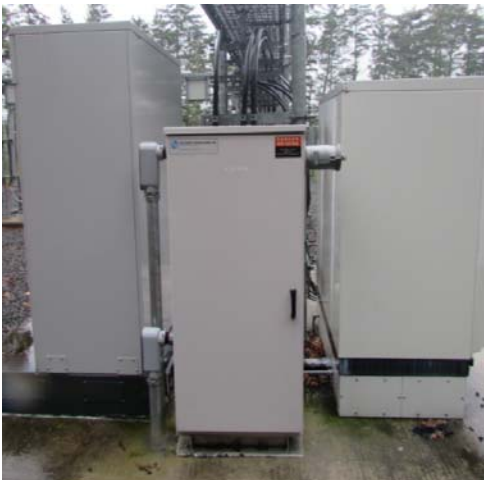
Equipment area with PPC & equipment cabinets.
