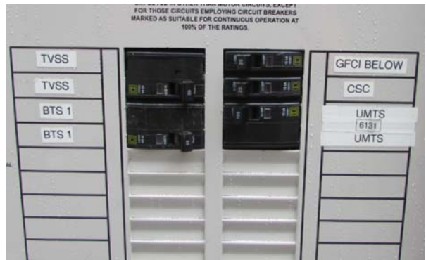
PPC breaker panel with new 100A breaker (Lower right breaker)
