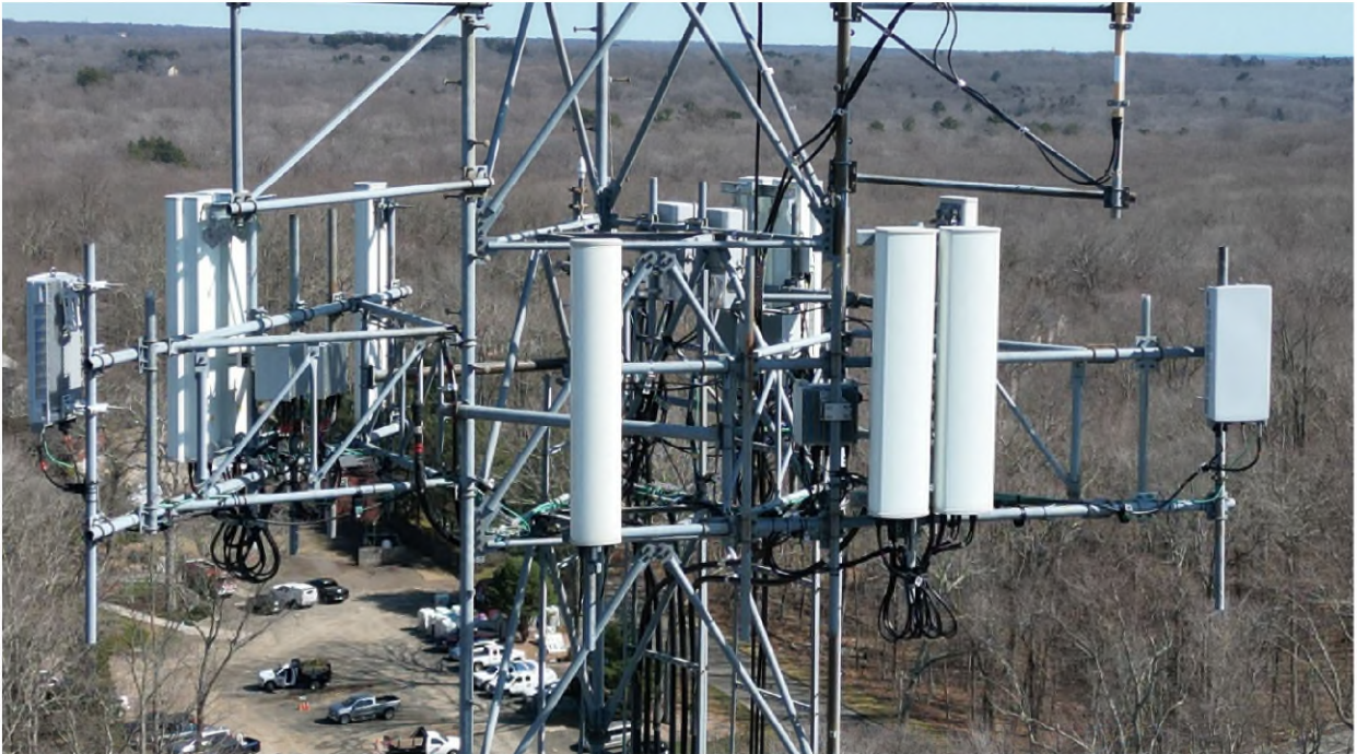
Fig. 3: Overall View of Antennas & Equipment (Gamma Sector)
