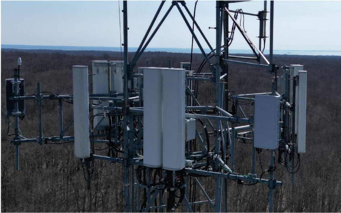
Fig. 1: Overall View of Antennas & Equipment (Alpha Sector)
