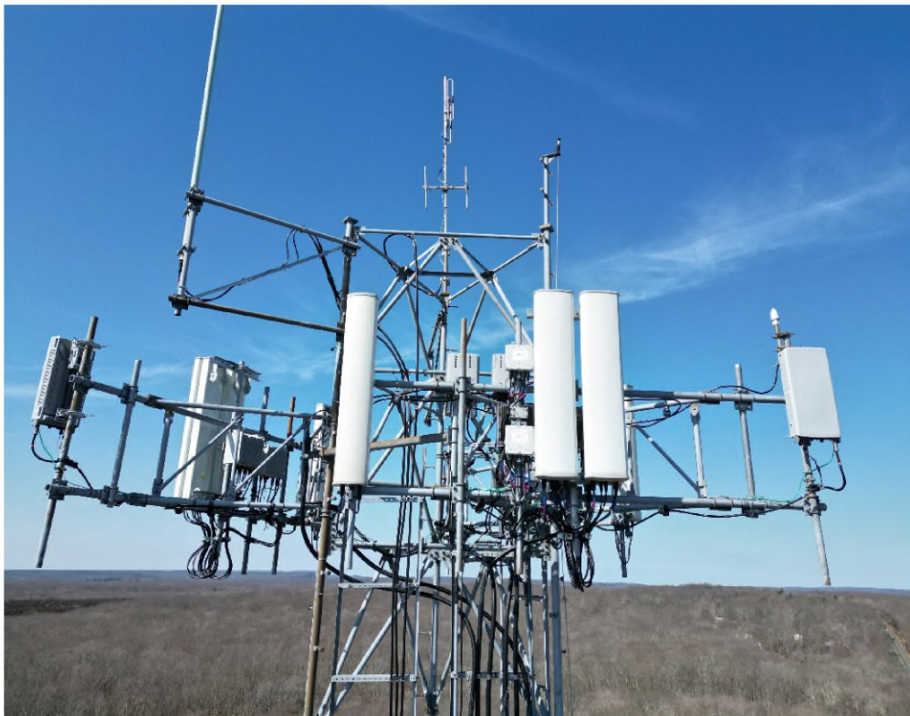
Fig. 2: Overall View of Antennas & Equipment (Beta Sector)
