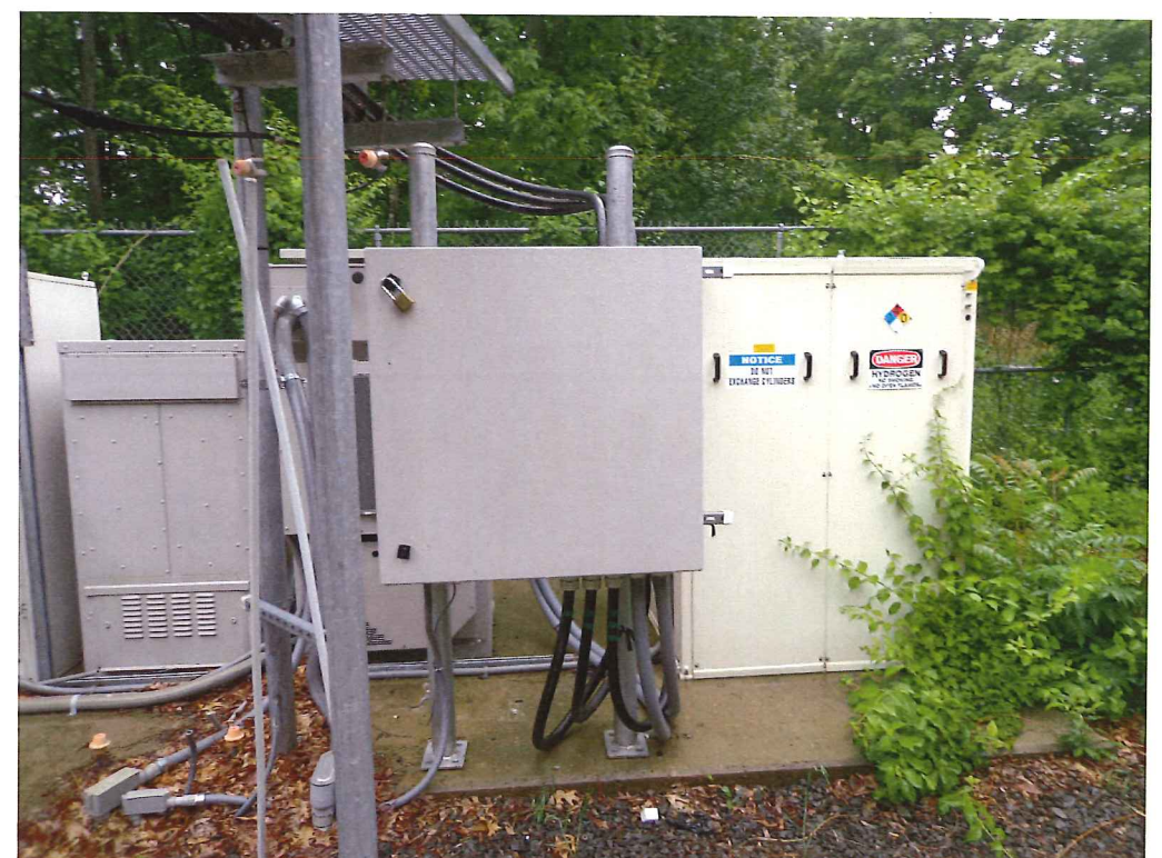
4 EXIST FIBER DISTRIBUTION BOX
