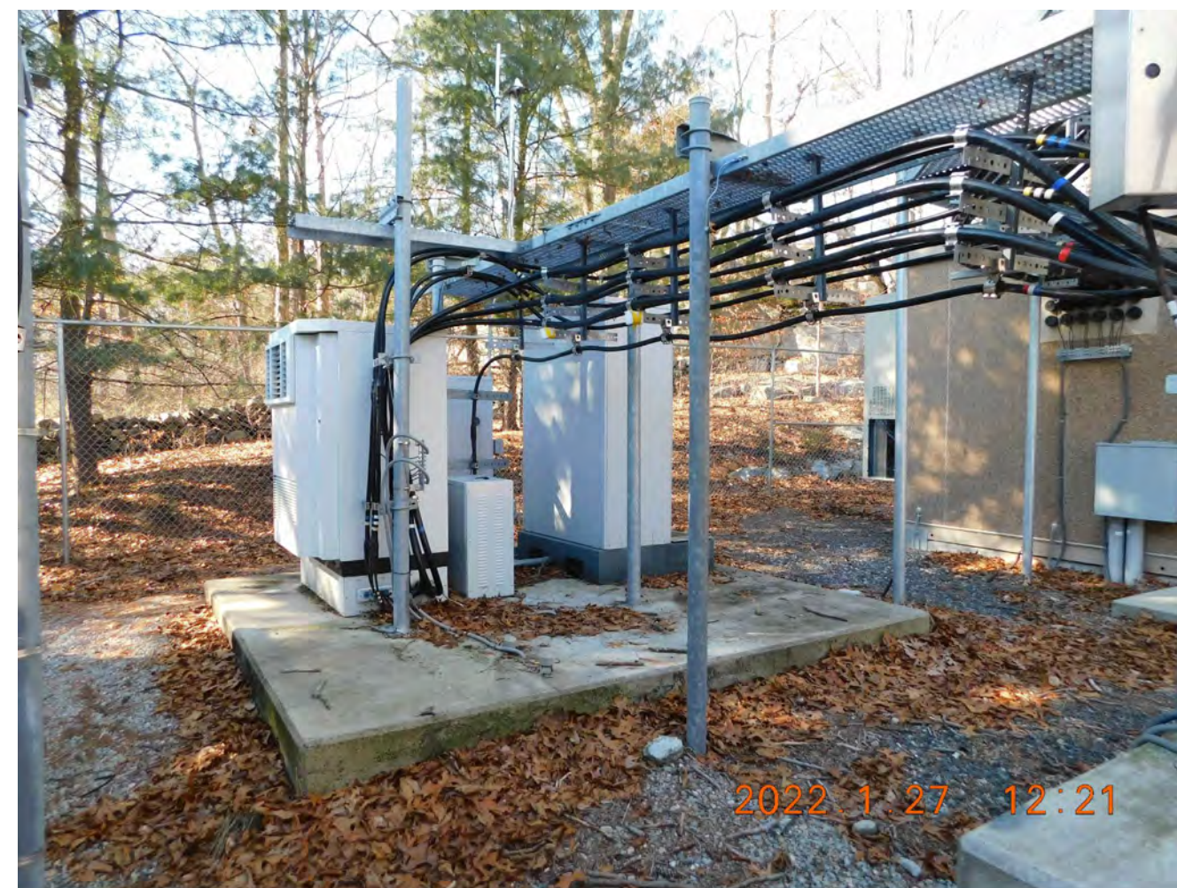
EXISTING EQUIPMENT PHOTO (2/A-1) SCALE: N.T.S.
