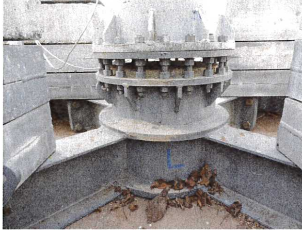
Image of existing \pm 85-ft tall AT&T temporary uni-pole tower ballast base frame and base plate assembly.
