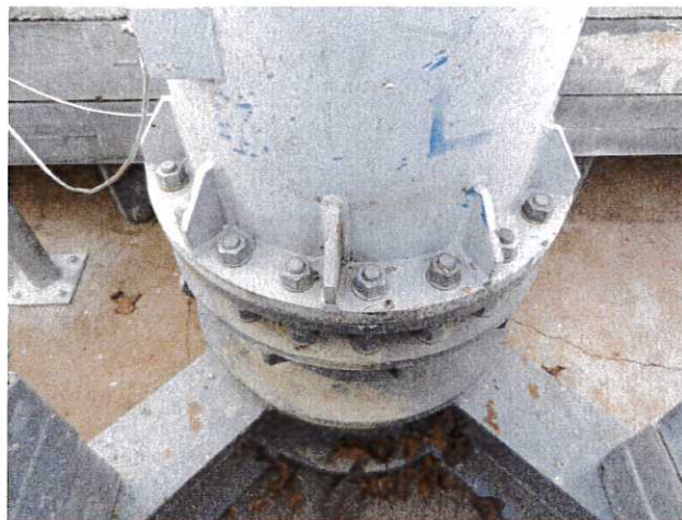
Image of existing \pm 85-ft tall AT&T temporary uni-pole tower ballast base frame and base plate assembly.
